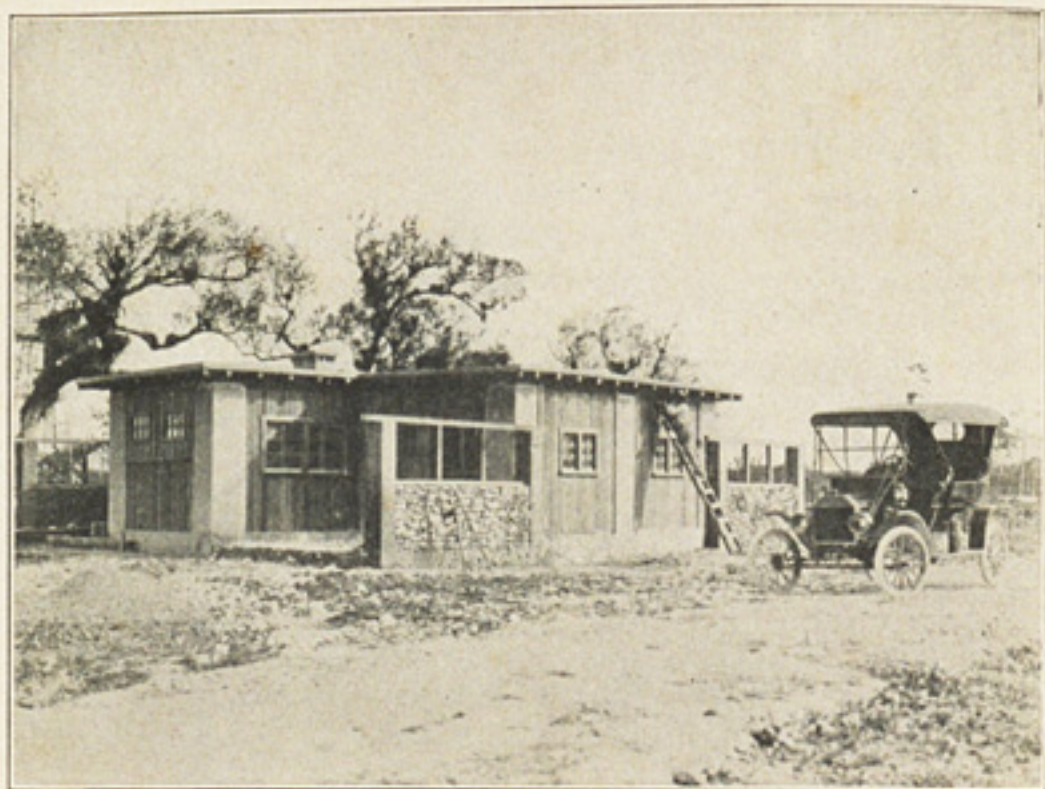
A UNIT HOUSE IN PROCESS OF CONSTRUCTION. CONCRETE ROOF AND CONCRETE FLOORS. THIS HOUSE CONSISTS OF THREE UNITS JOINED TOGETHER ON A TRIANGULAR LOT. VIEW FROM SOUTHWEST. (PHOTO BY KAUFMAN, MIAMI, FLA.)
