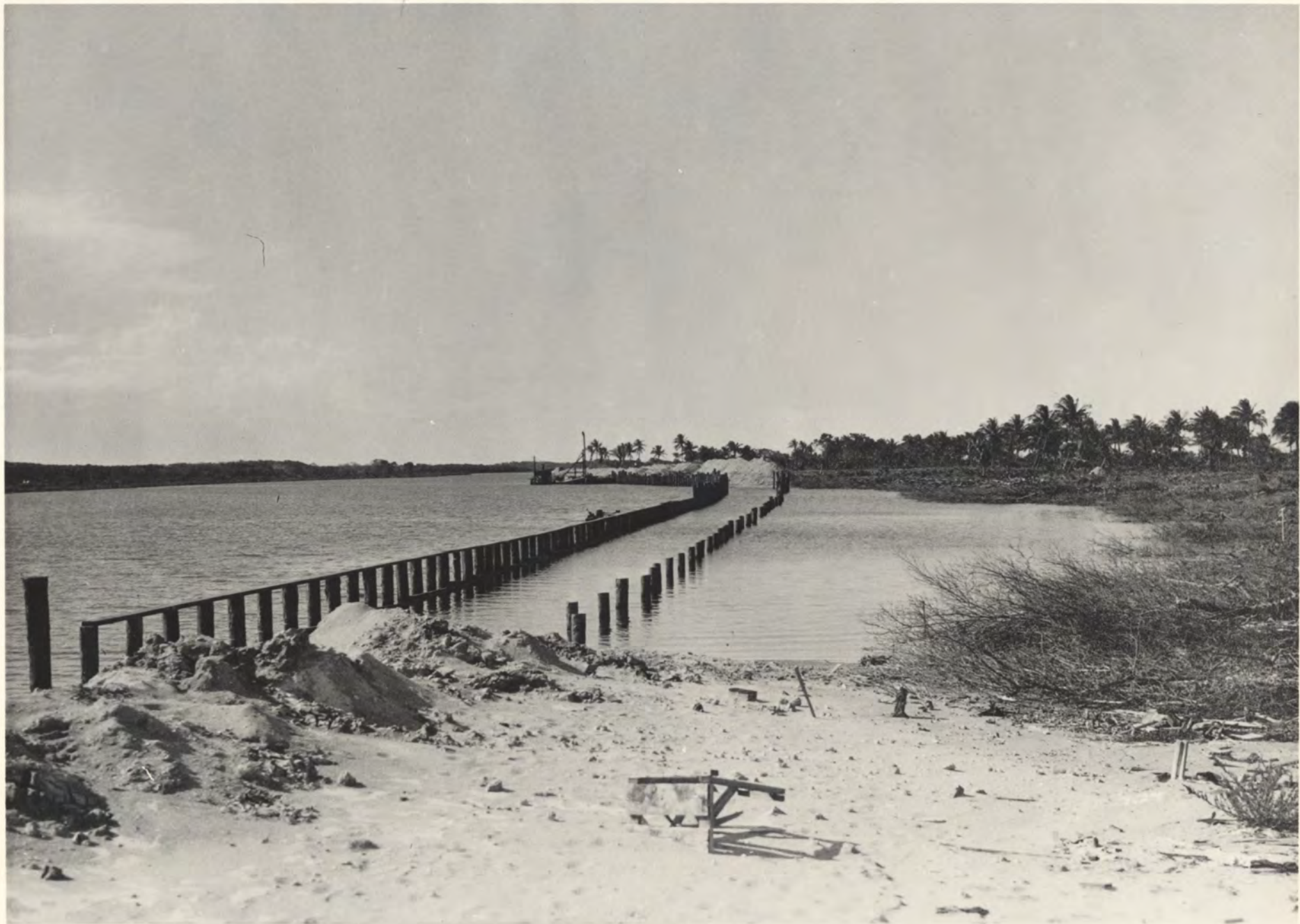
22-13. 1920—The bulkhead under construction on the east side of Indian Creek, looking north from about Fiftieth Street.
