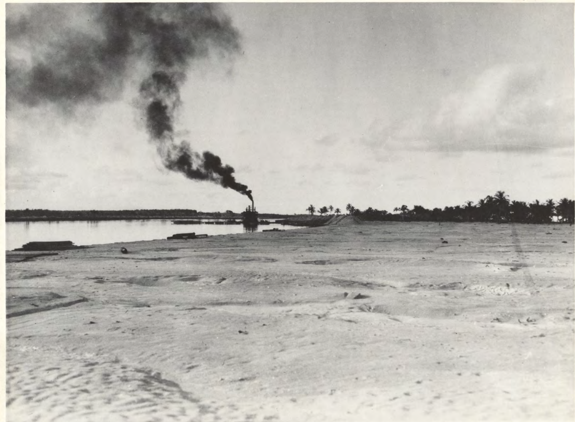
25-13. Sept. 13, 1920—East side of Indian Creek, about Fiftieth Street, showing the dredge at work on the fill..
