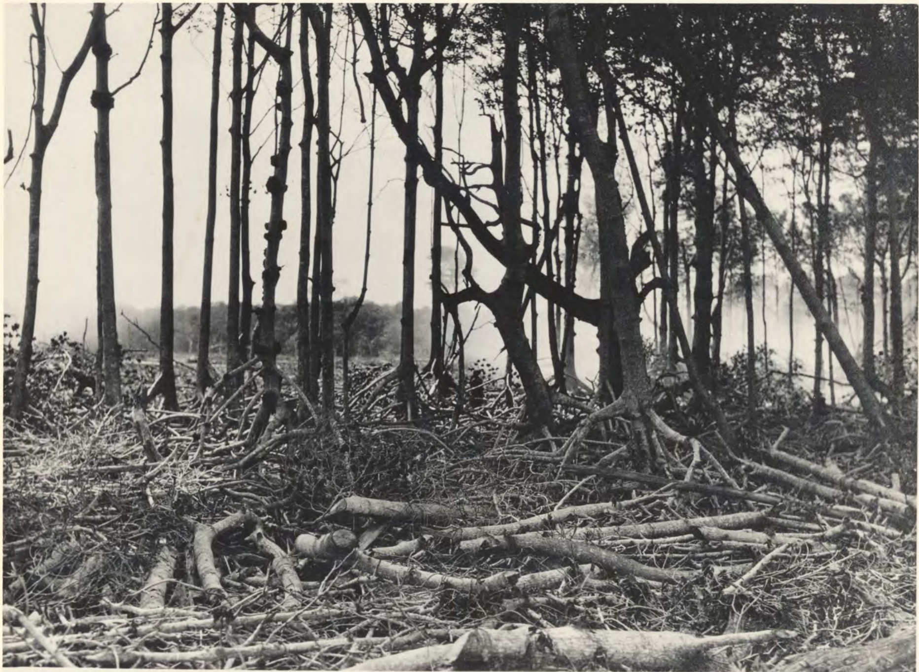
19-13. 1920—A section through the mangrove forest in the north Bay Shore section during clearing operations.
