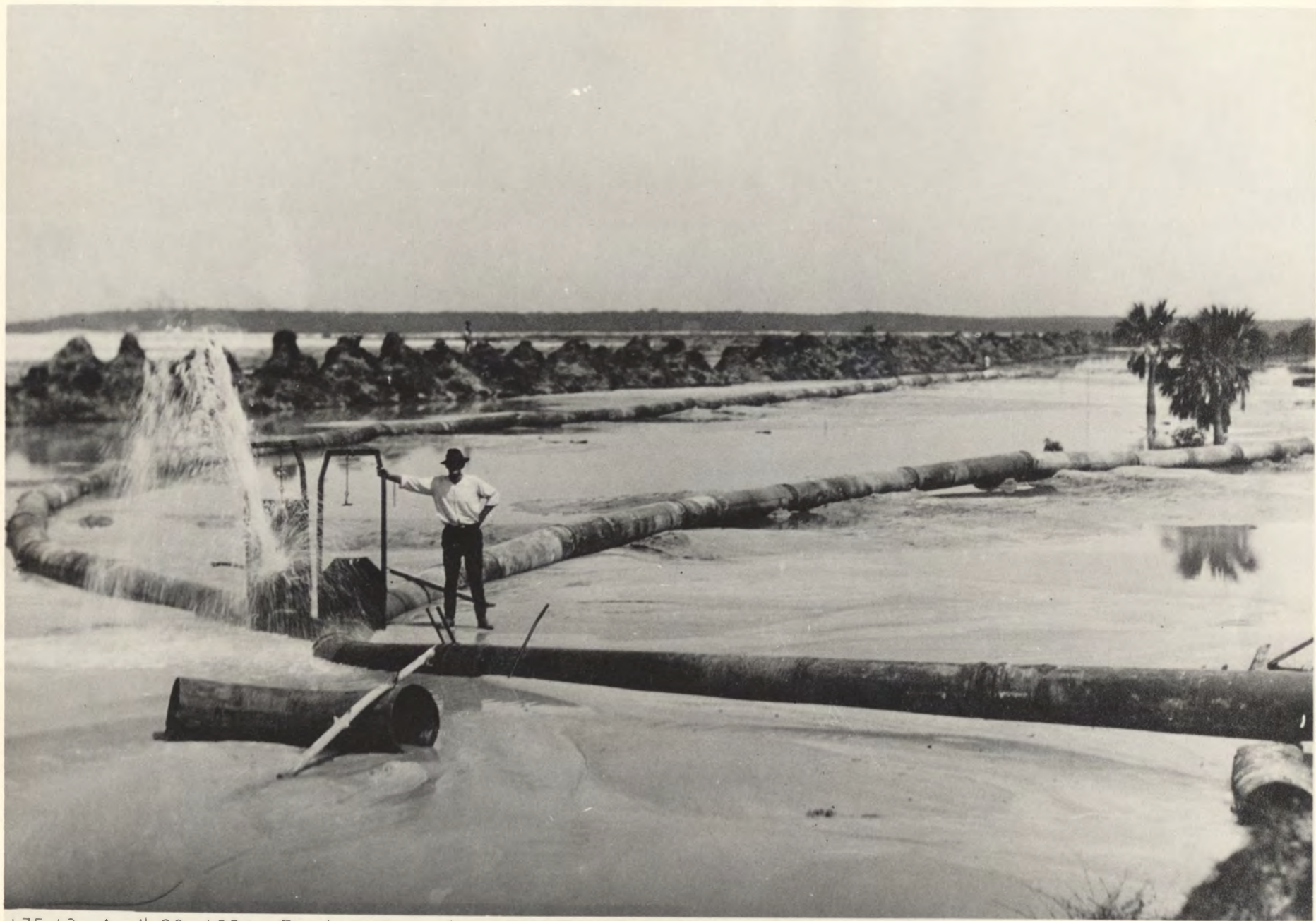
175-13. April 28, 1924—Dredge pipes along Pine Tree Drive and LaGorce Drive at about Fifty-second Street. The piles of dirt are top-soil which was spread on top of the fill after it had settled and dried.
