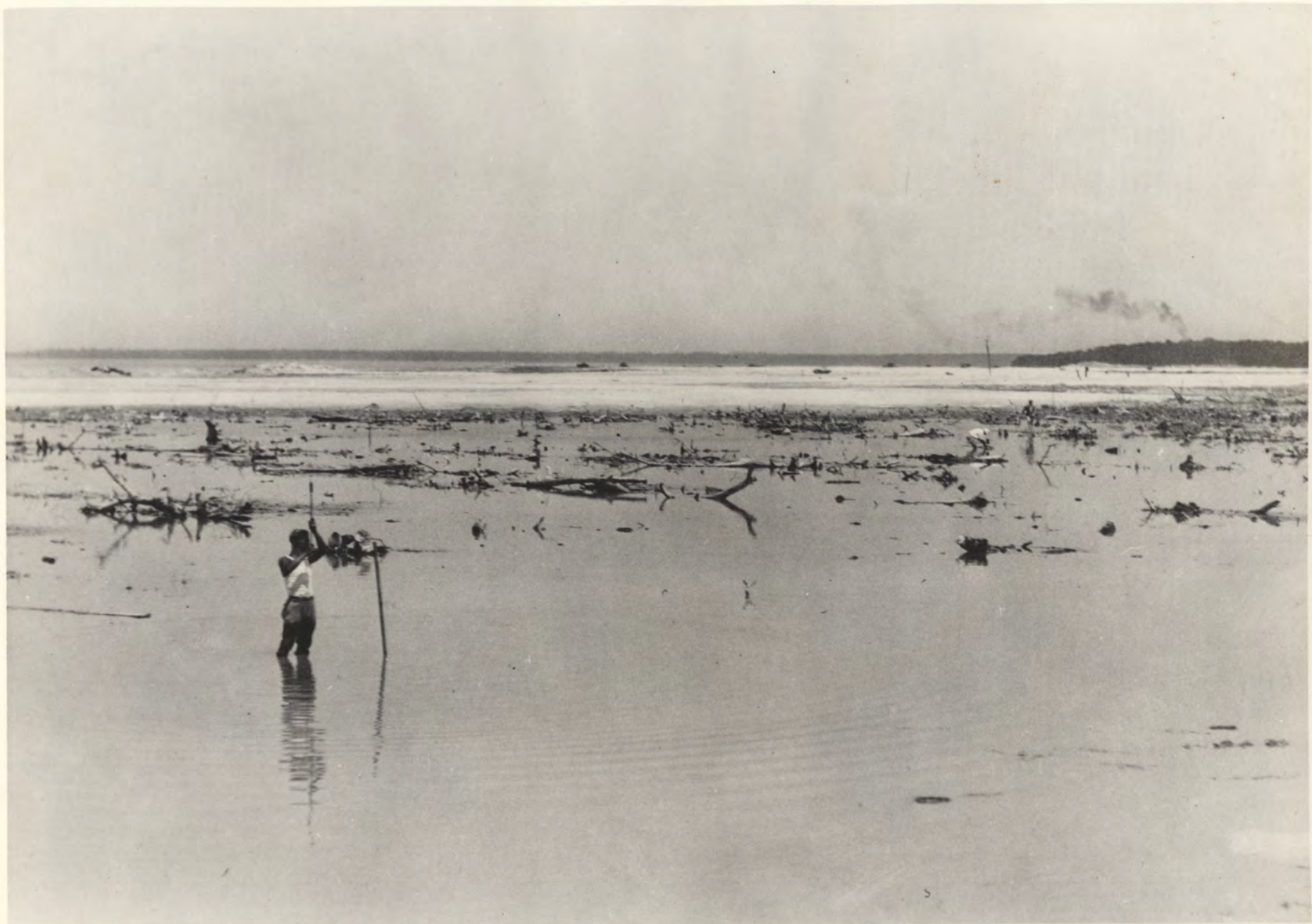
179-13. 1924—Surveyor driving leveling stakes for the fill in the North Bay Shore section, about Alton Road and Fiftieth Street.
