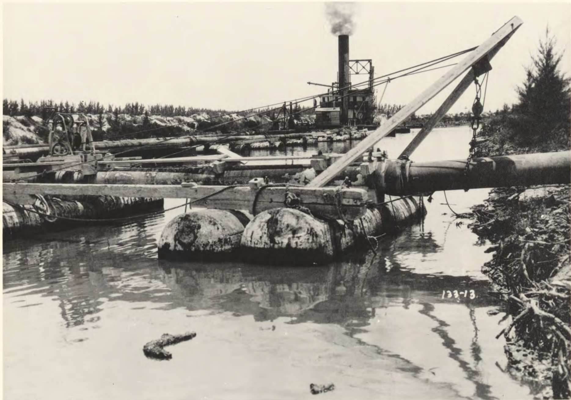
133-13. 1923—Discharge end of the suction dredge, showing the floats supporting the discharge pipes. The dredge is near Sunset Lake.
