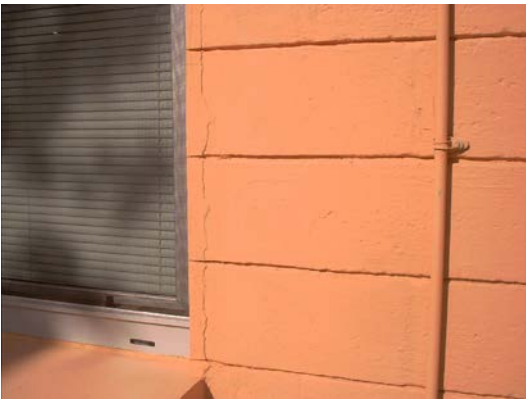
Exterior cracks surrounding the office window area at concession stand building at Virginia Key Beach Park
