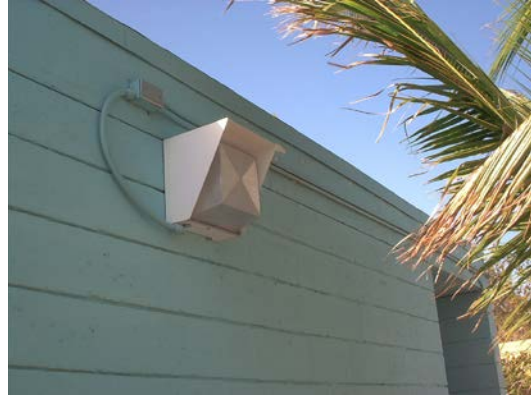
Exterior lighting does not meet codes for protected sea turtle nesting on bathhouse at Virginia Key Beach Park
