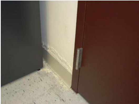
Baseboard water damage in concession stand building at Virginia Key Beach Park
