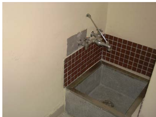
Baseboard water damage in janitor closet in concession stand building at Virginia Key Beach Park
