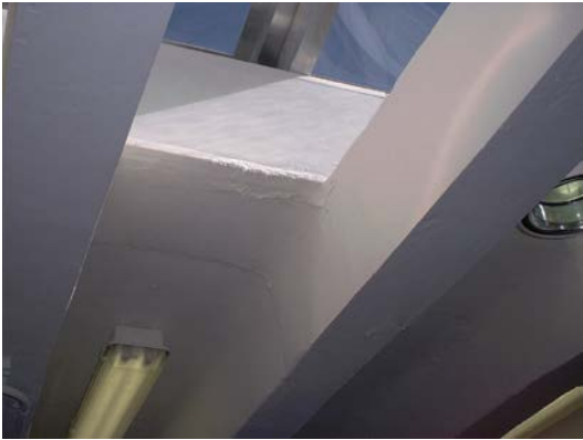
Water damage near ceiling of men's restroom in bathhouse at Virginia Key Beach Park
