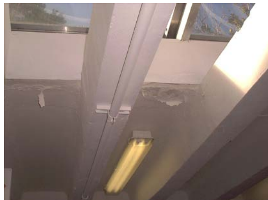
Water damage near ceiling of women's restroom in bathhouse at Virginia Key Beach Park
