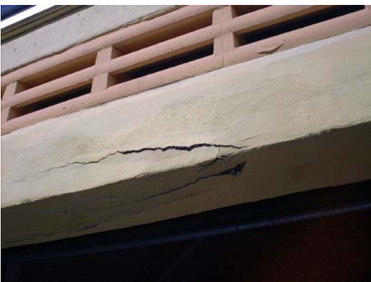
Wall on Northern end of the carousel building cracking
