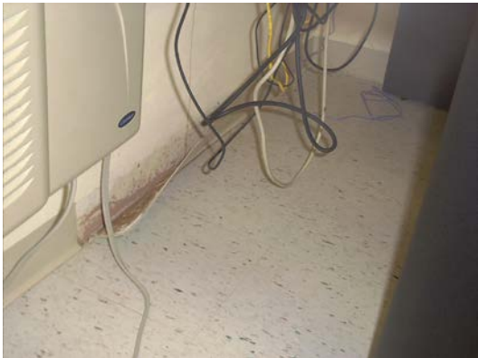
Baseboard water damage in concession stand building at Virginia Key Beach Park
