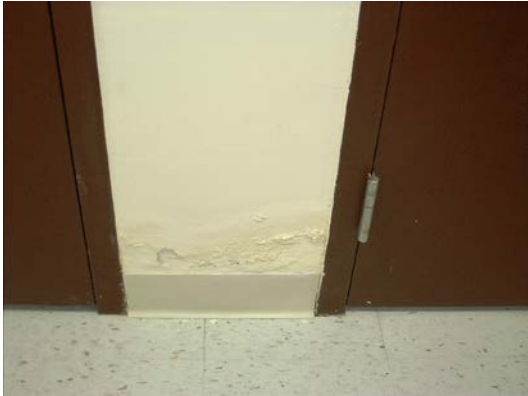
Baseboard water damage in concession stand building at Virginia Key Beach Park
