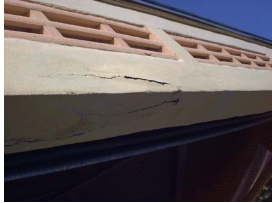
Wall on Northern end of the carousel building cracking
