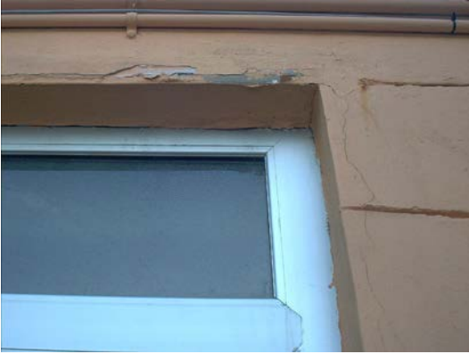
Close up of exterior cracks surrounding the restroom window of the concession stand building
