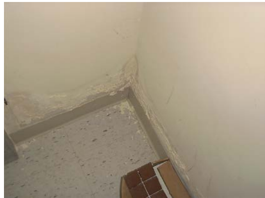
Baseboard water damage in janitor closet in concession stand building at Virginia Key Beach Park
