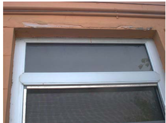
Exterior cracks surrounding the restroom window of the concession stand building
