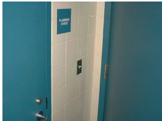
Light switch installed behind the door of men's handicapped restroom in bathhouse at Virginia Key Beach Park
