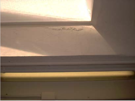
Water damage near ceiling of women's restroom in bathhouse at Virginia Key Beach Park
