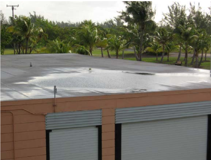
A tour of the roof with Jorge, Chris (CW Construction) and a roofing contractor uncovered standing water. (See Above)
