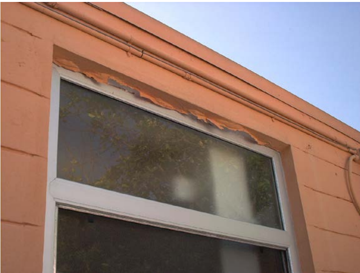
Concrete damage around windows on the concession building – Northwest side. (See above)
