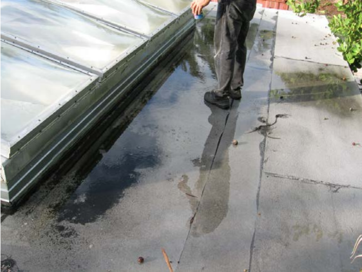
A tour of the roof with Jorge, Chris (CW Construction) and a roofing contractor uncovered standing water. (See Above)
