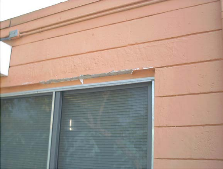
Concrete damage around windows on the concession building – Southwest side. (See above)
