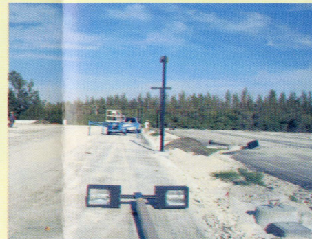
* Parking lot light fixtures: CW Construction completes the installation of light fixtures on Historic Virginia Key Beach Park
