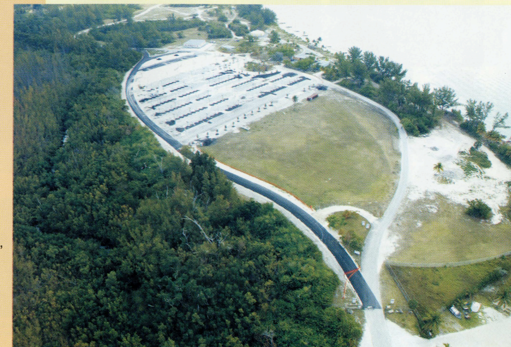
* CW & Metric Staff: Christopher North, CW Construction and Maria Elena Mariner, Metric Engineering are the on-site supervision that coordinate with the Trust to make the parking lot project meet its deadlines.
