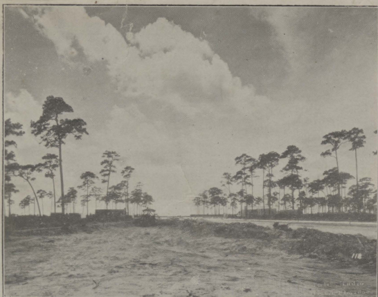
ONE of the giant steam shovels at Fulford By-the-Sea is shown here cutting down the final grade on Fulford Boulevard. It stands today just one block away from the Royal Glade Canal. This boulevard will be completed and ready for asphaltting within the next few weeks.
