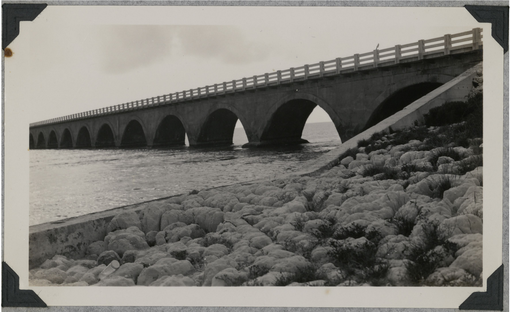
View of east end of Long Key Viaduct. Note the marl fill in foreground which would require top dressing before area could be used for parking.
