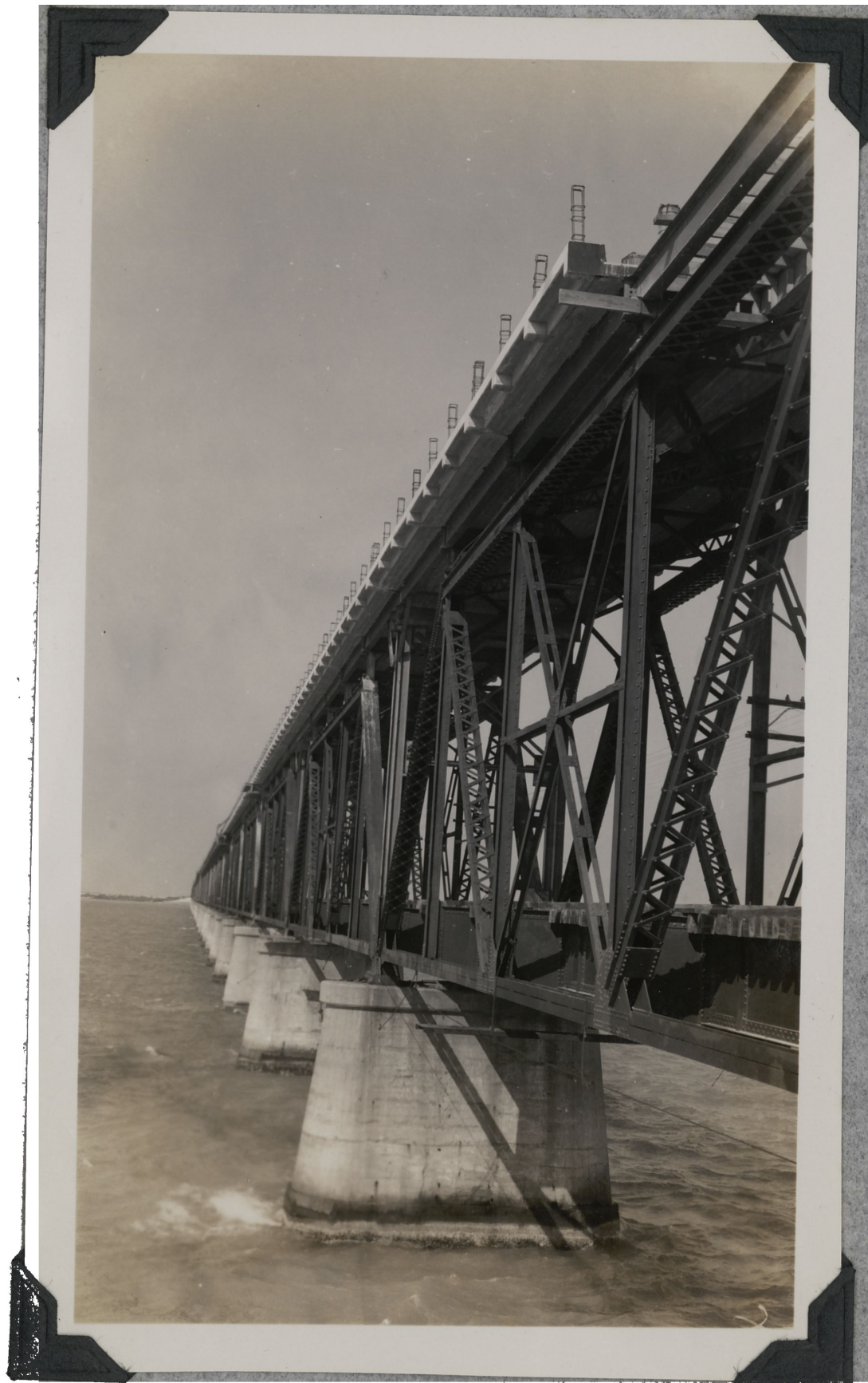
Close up view showing upper and lower decks of the West Switzerland - Bahia Honda Bridge
