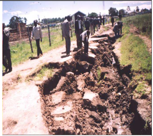
Figure 5. 7. Gully formation and soil erosion along access road to Bomet Town, upstream of 1LA03.
