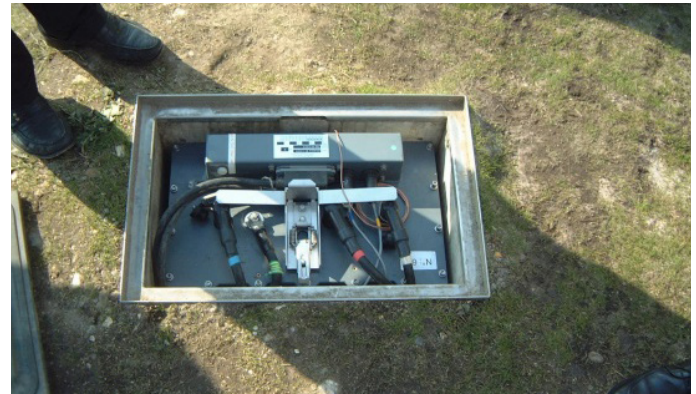
FIGURE 4.30: IN-GROUND CONTACTOR BOX
