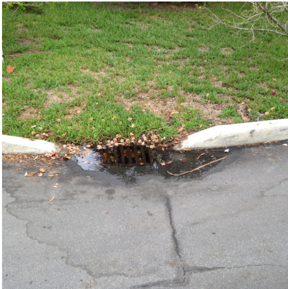
Figure 1 - Catch Basin on Mola Drive with Tide Water Rising.
