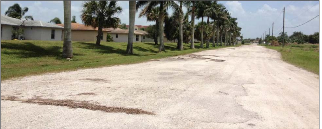
Figure 3-6: An existing Belle Glade street is filled with potholes and is difficult to navigate
