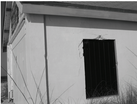
Figure 145. Example of damage to concrete walls at south elevation.
