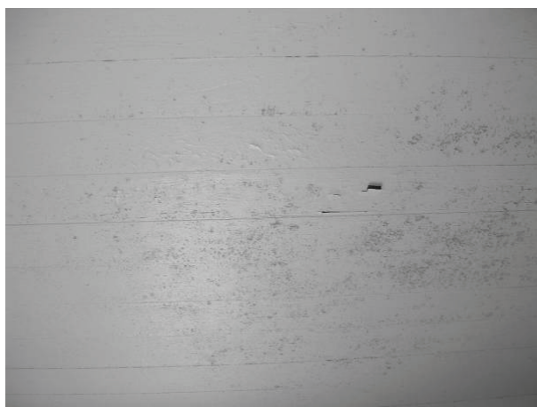
Figure 116. Deteriorated paint finish at the second floor ceiling.
