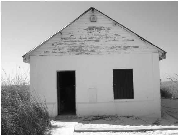
Figure 136. East elevation of Boat House. 134. Horizontal crack in eave fascia at east elevation.
