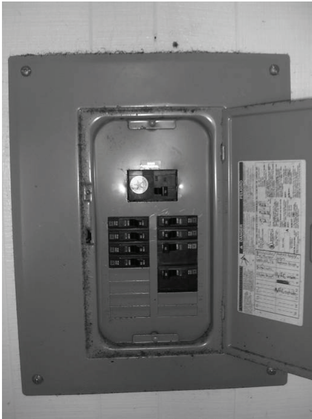
Figure 118. Close-up of eight-circuit distribution panel at Kitchen Building.
