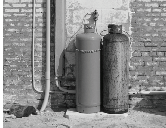
Figure 87. New and rusted propane gas tanks at west elevation.
