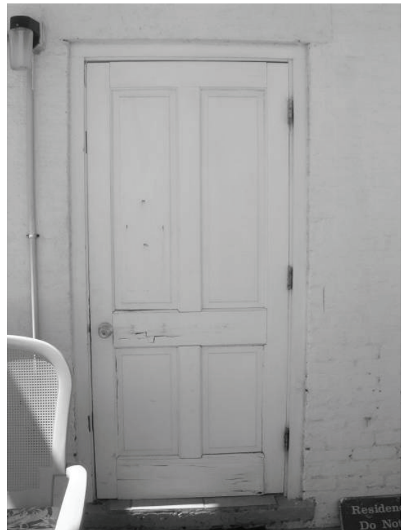
Figure 94. Exterior face of front door with cracking.
