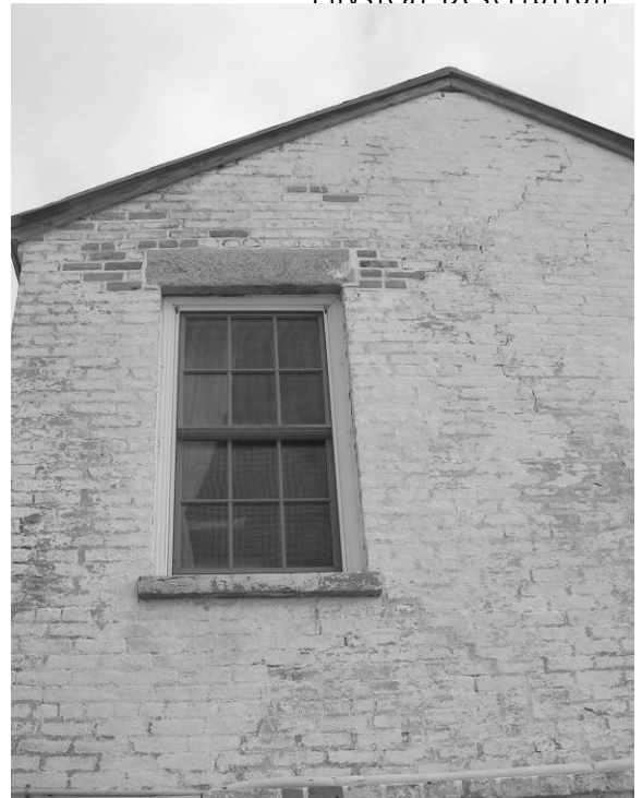
Figure 93. Several cracks emanate from a central location. It is possible that this damage may have been caused by a tree or other projectile hitting the building during a storm.
