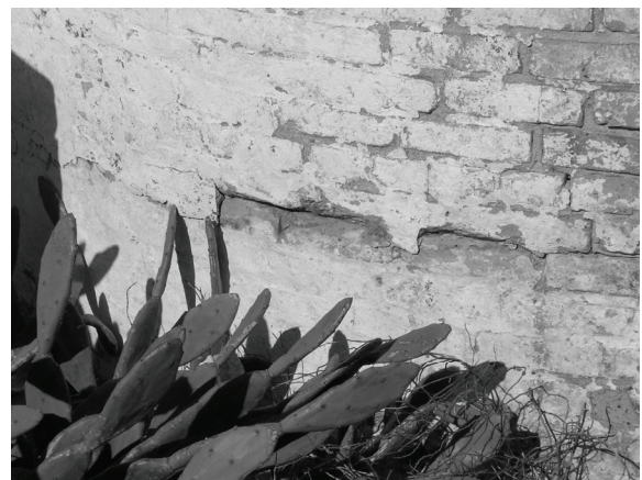
Figure 126. Deteriorated mortar joints and bricks at lower courses of south brick cistern.
