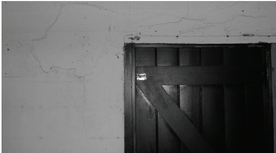
Figure 152. Example of damage to interior face of concrete walls.
