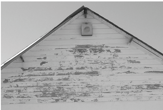
Figure 137. Weathered novelty siding in gable end at east elevation.
