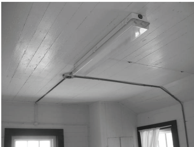
Figure 119. Fluorescent light fixture and rigid metal conduit at second floor.
