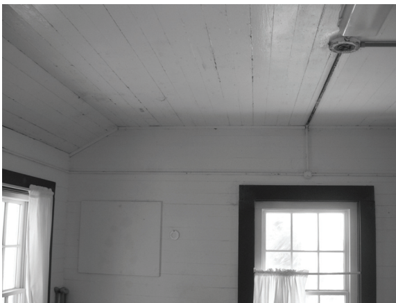
Figure 109. View of horizontal tongue and groove walls at second floor – facing northeast.
