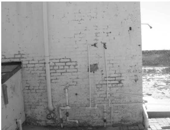
Figure 123. Plumbing pipes at north elevation.
