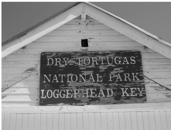
Figure 139. Deteriorated paint finish of novelty siding and signage at west elevation.
