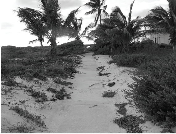
Figure 160. Damaged concrete walkway extending west toward Kitchen Building.
