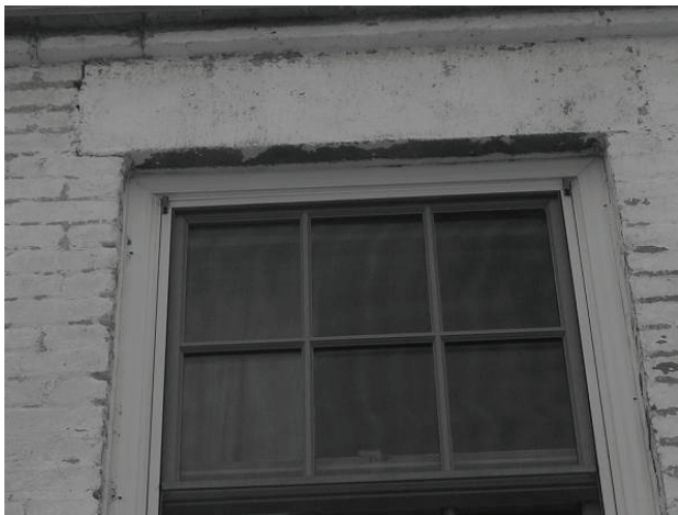
Figure 96. Typical condition of painted concrete window lintels.
