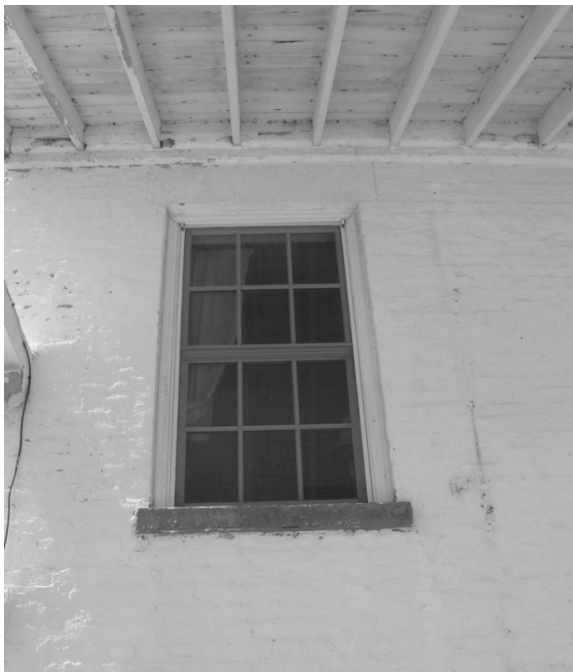
Figure 84. Deteriorated mortar at cornice on east elevation.
