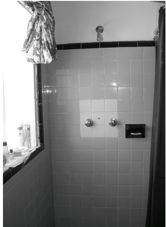
Figure 106. View of ceramic tile at shower and window. Damaged tile at window edge.
