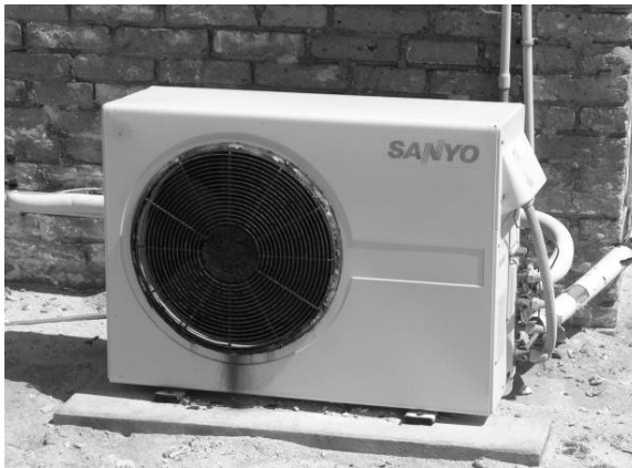
Figure 122. Air compressor at west elevation.
