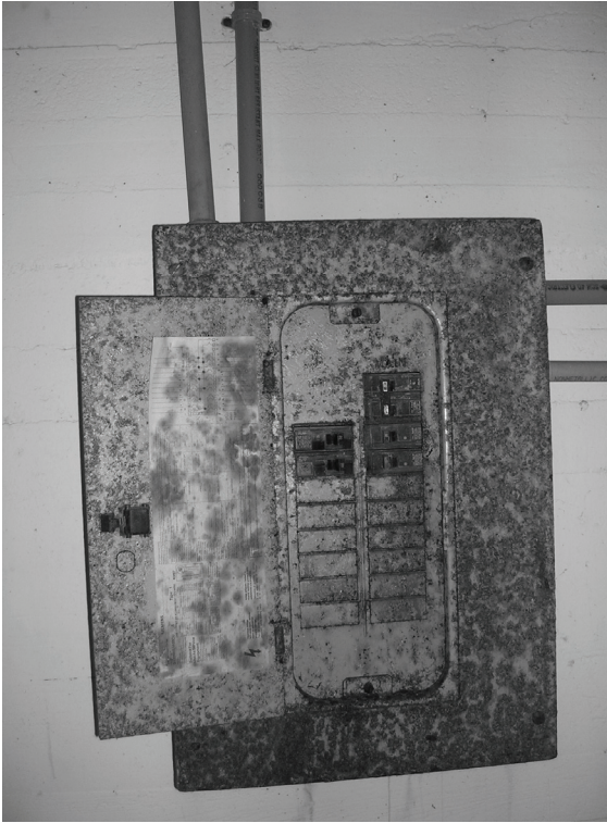
Figure 154. Close-up of six-circuit distribution panel in corroded condition.
