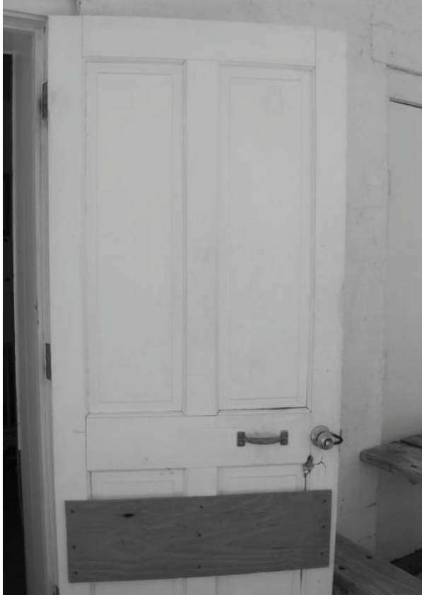
Figure 95. Interior face of front door with cracks and ¼” plywood brace.
