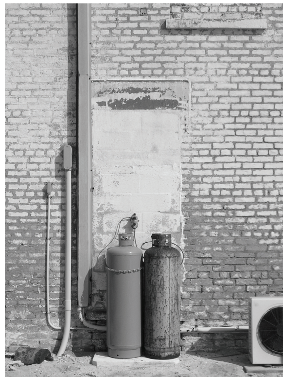
Figure 120. Propane gas tanks at west elevation.
