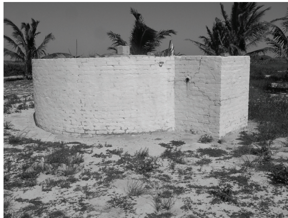
Figure 128. Cracks at intake box of south cistern.
