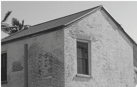
Figure 81. Damaged flashing at rake board.
