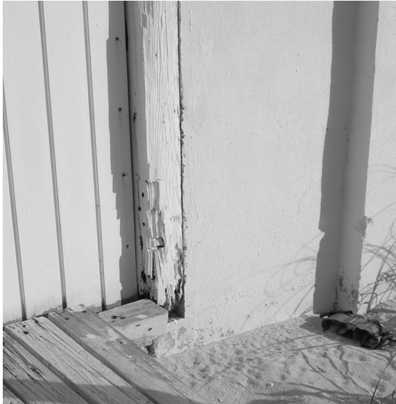
Figure 141. Damaged vertical framing at west elevation.
