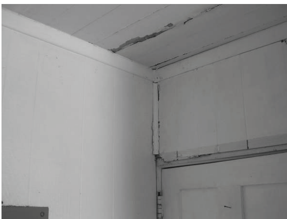
Figure 103. Deteriorate ceiling finish and wall boards above bathroom door.
