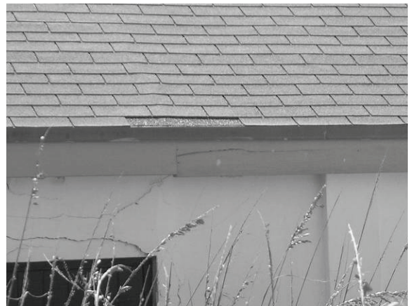
Figure 134. Horizontal crack in eave fascia at east elevation.
