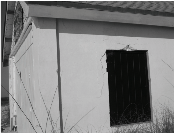
Figure 145. Example of damage to concrete walls at south elevation.
