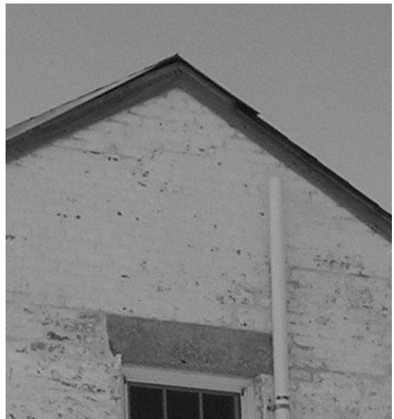
Figure 89. Areas of previous repairs.
