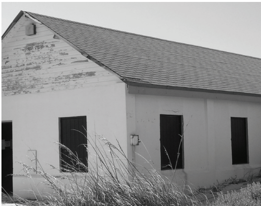
Figure 153. Metal switch box at northeast corner of building.
