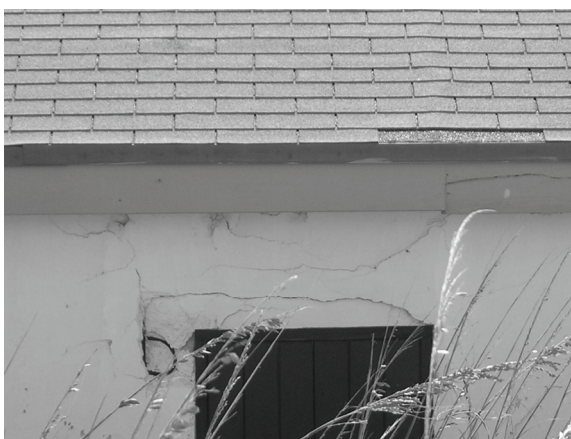
Figure 143. Example of damage to concrete walls at north elevation.
