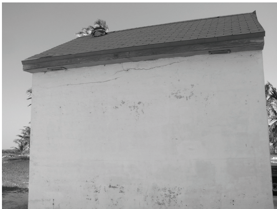
Figure 157. Cracks in mortar joints at the north elevation of New Oil House.
