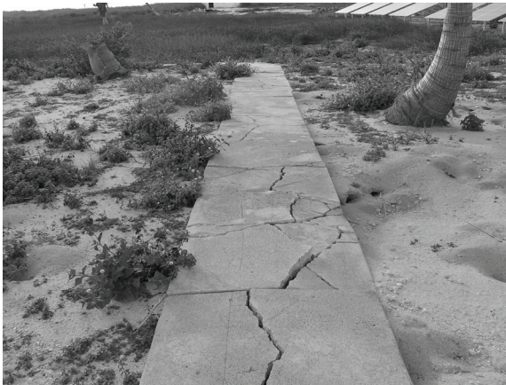
Figure 161. Damaged concrete walkway extending west, with the solar array to the north.
