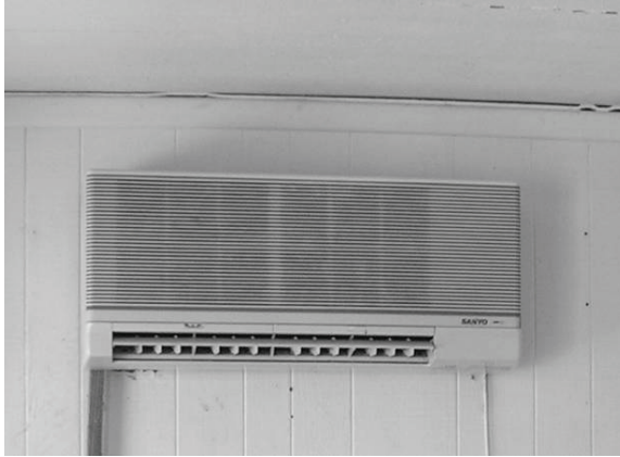
Figure 121. Sanyo cooling unit on first floor.
