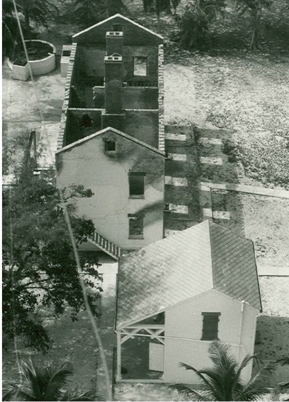
Figure 67. Undated view of fire damaged Keeper's Dwelling.
