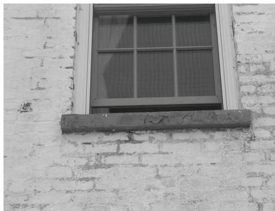
Figure 97. Typical condition of painted concrete window sills.
