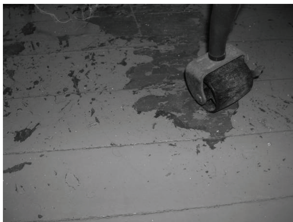
Figure 117. Deteriorated floor finish at the floor on second floor.
