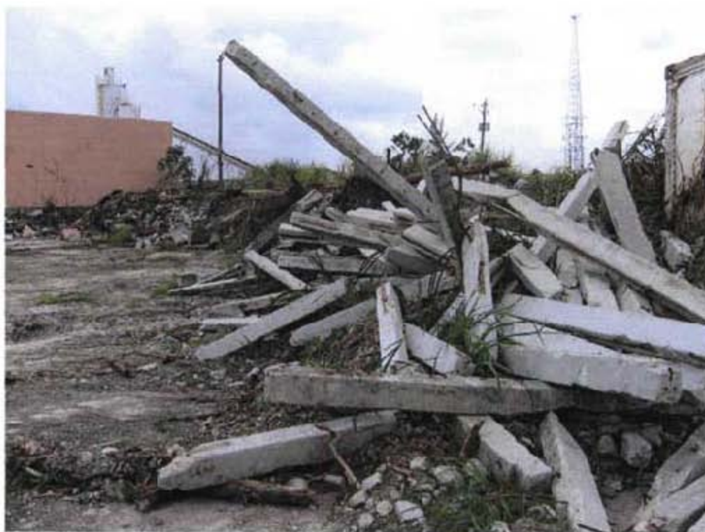
Debris on Payne parcel and view of buildings on NW 109 th Street.
