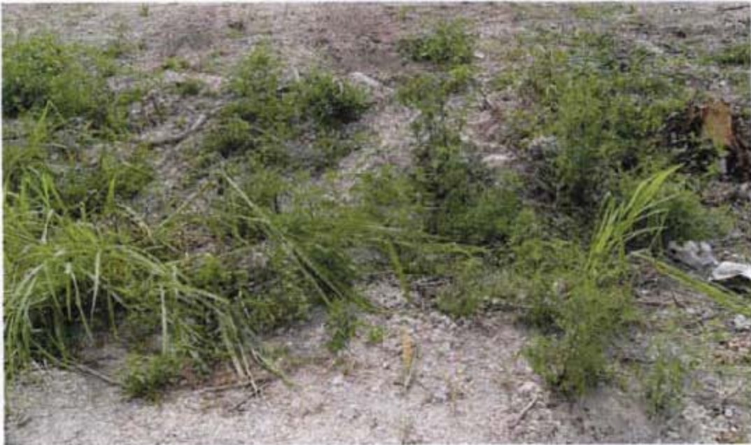
Vegetation growing in original drainage collar around monolith.
