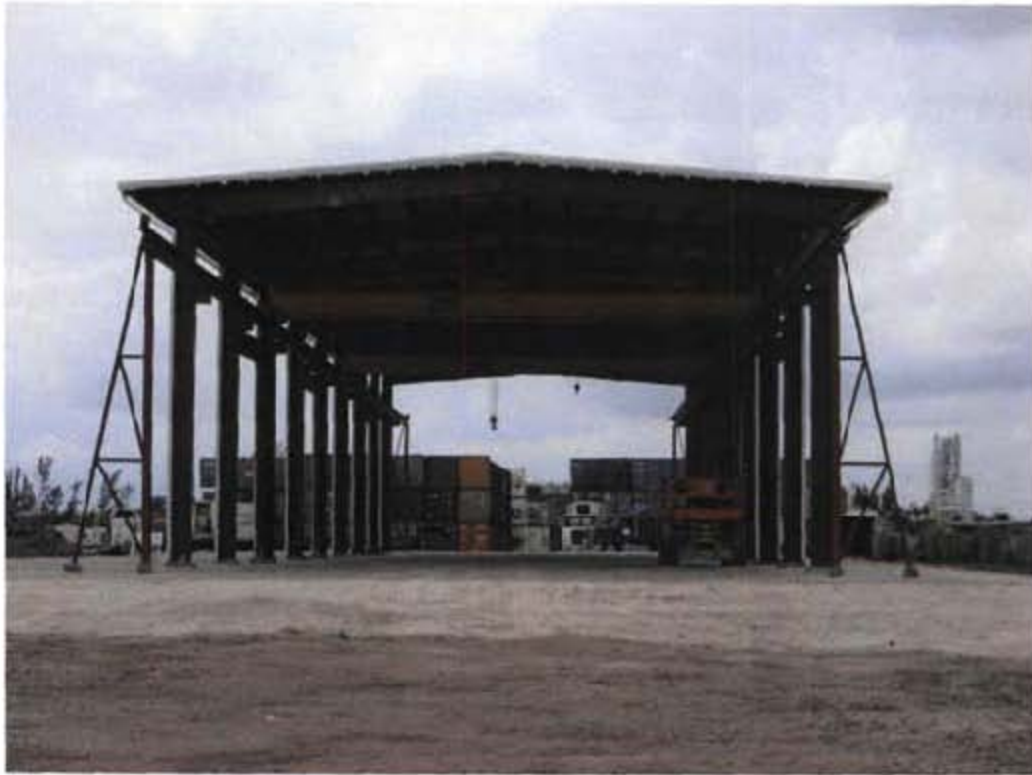
Building under construction on Payne parcel monolith will be a concrete products facility.
