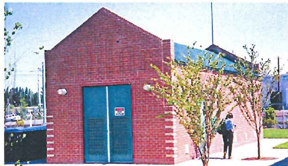
Portland's Tri-Met system employs visually interesting architectural treatments for power substation structures
