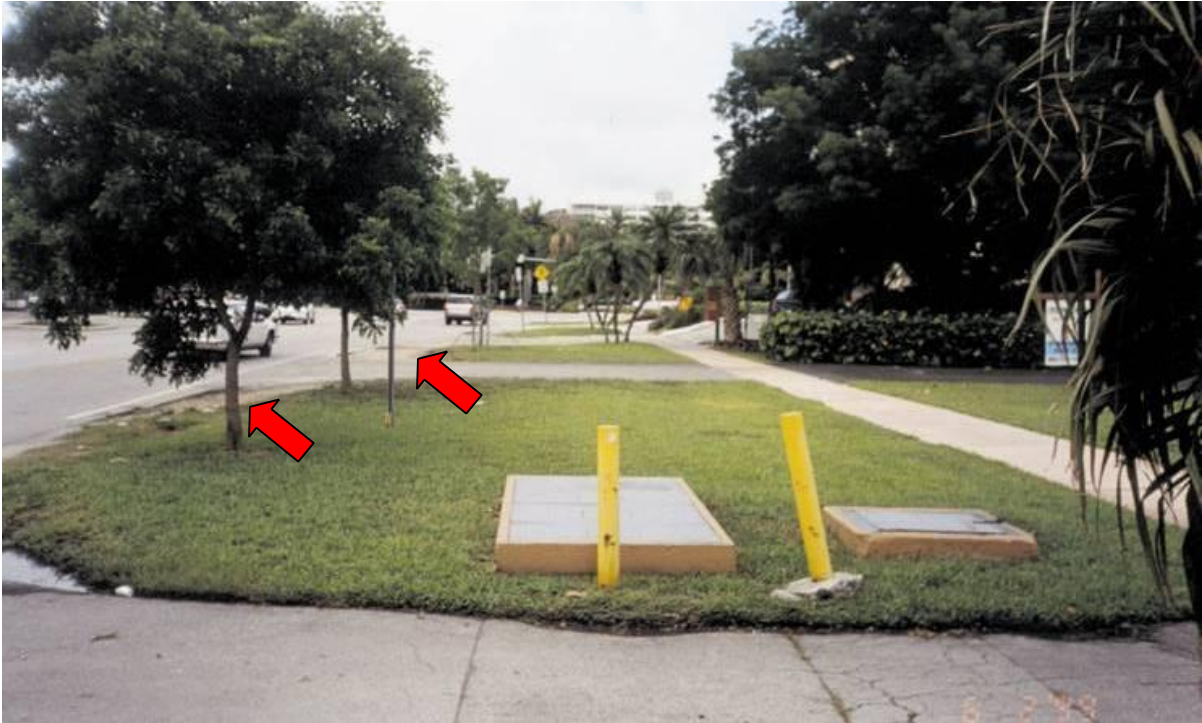
Swale Damage due to Vehicles Driving on Shoulder
