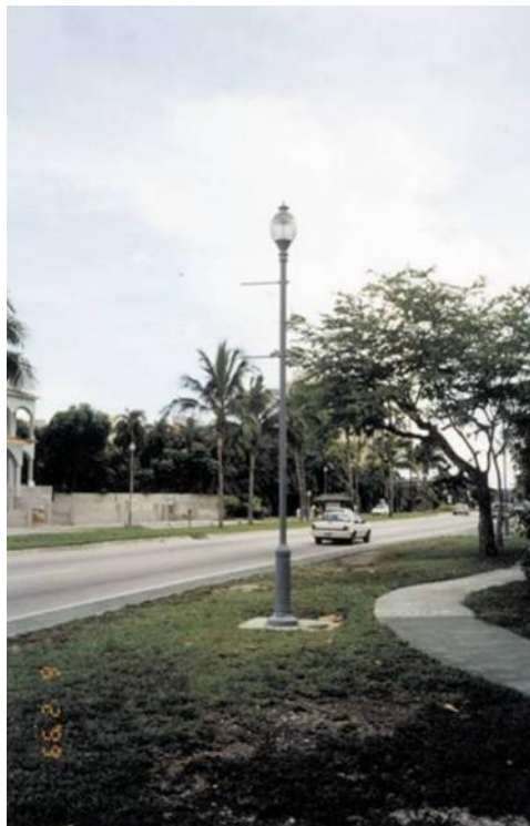
Existing Street Lights
