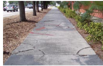
Deteriorating pavement conditions
