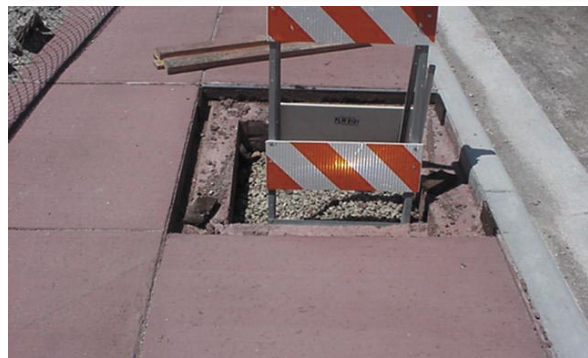
Step 2 - Pouring sidewalk directly over the compacted structural soil. The tree pits is then dug-out for the root ball.
