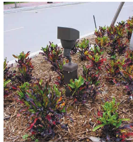
Similar fixture placed on metal stanchion in a planted median.
