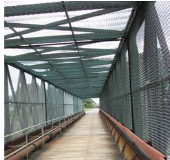
Utility lines interfere with trail width
