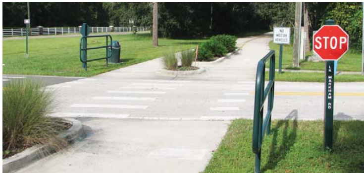
Seminole-Wekiva Trail, at-grade crossing with raised landscape median and bar lean rail
