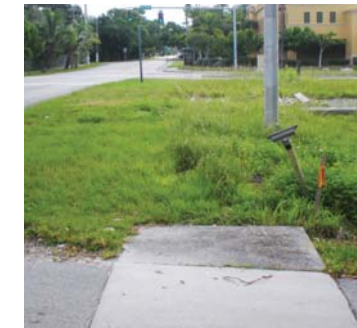
Example of disconnected sidewalk near SW 80th St.
