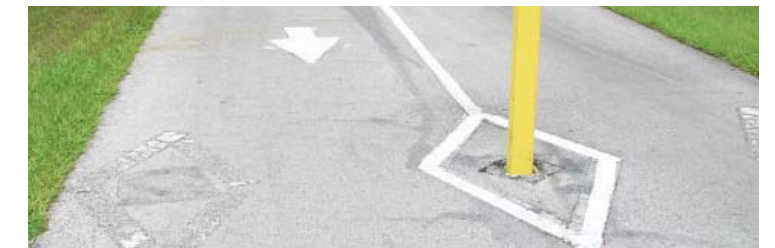
Example of removed bollards along West Orange Trail
