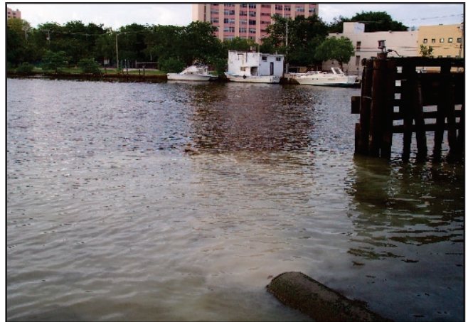
A stormwater outfall directly into the Miami River
