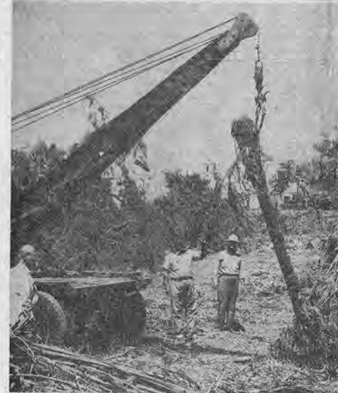
Leveling of plot for Coral Gables War Memorial-Youth Center was progressing rapidly this week. At left forefront Harry W. Morgenthauer Jr., president of the association, supervises one branch of the clearing project.
