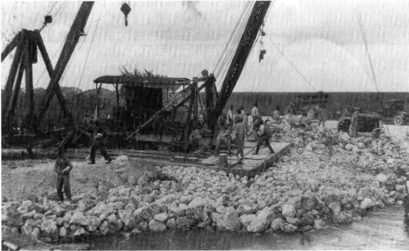
A dredge with a team of workers creating a drainage canal. HASF 85-226-4.
