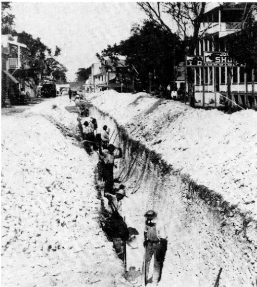
A view of the sewer ditch; looking north on Miami Avenue at today’s S.E. 3rd Street.
