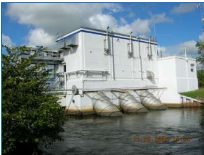
Figure 38 - S-13 Pump station located on C-11 canal at US441 and Orange Drive in Davie, FL. It has a rated capacity of 540 cfs, and can pump approximately 14.5 million gallons per hour (SFWMD, 2007).
