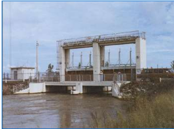
Figure 51 - Salinity structures control flooding by releasing primary canal water to tide when necessary. They are also used to maintain elevated canal levels for stormwater storage and to recharge aquifers and control saltwater intrusion. (SFWMMD)
