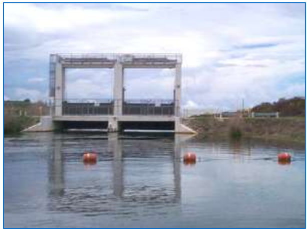
Figure 37 – Typical coastal flood/salinity control structure of the sluice gate type. (SFWMD)
