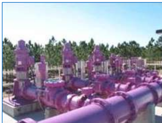
Figure 63 - Piping used for distribution of reclaimed wastewater is colored purple to distinguish it from potable water pipes. (SFWMD)
