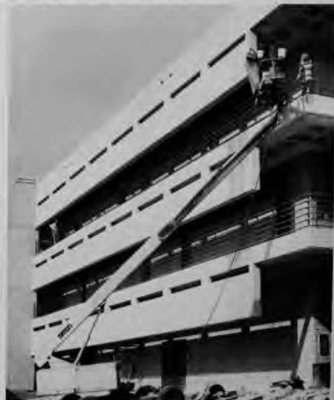
With a little help from a mechanical friend, the building is finished.
