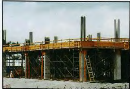
Near the Graham Center, the Health Sciences building was under construction. Photo By Jose Otero
