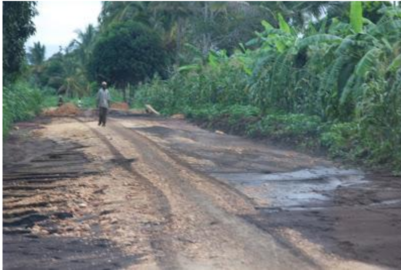
Figure 16: Mass movement of soils across a roadway in the "m" area
