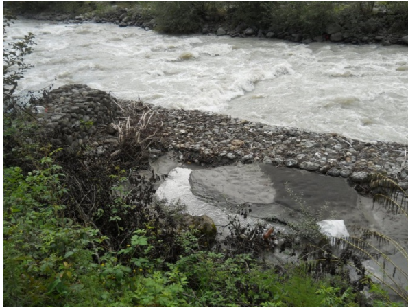
Pic. 4. The village Lagvanta. The Sakaura River. Unfinished bank protection structure
