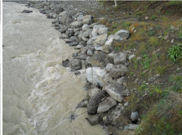
Pic. 5. The village Lagvanta. The Sakaura River. Destroyed rockfill berm
