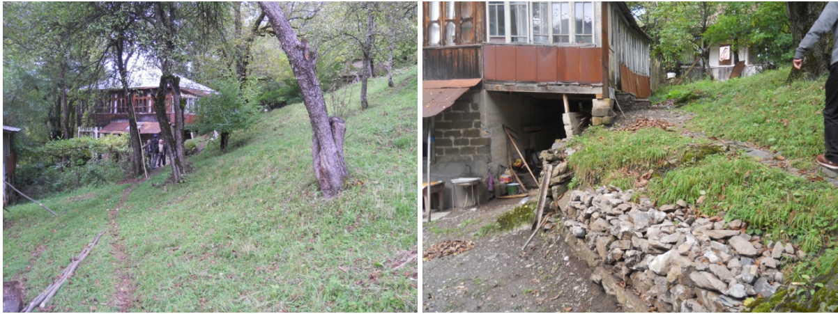
Pic. 13, 14. The village Khideshlebi. Residential houses damaged as a result of landslide activity
