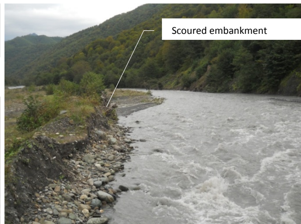
Pic. 3. The village Likheti. Scoured rock-fill embankment on the right bank of the Lukhunistskali River
