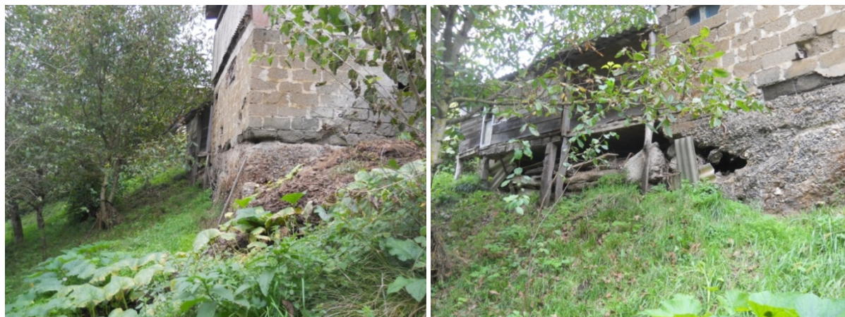
Pic. 13, 14. The village Abari. Buildings damages by landslides
