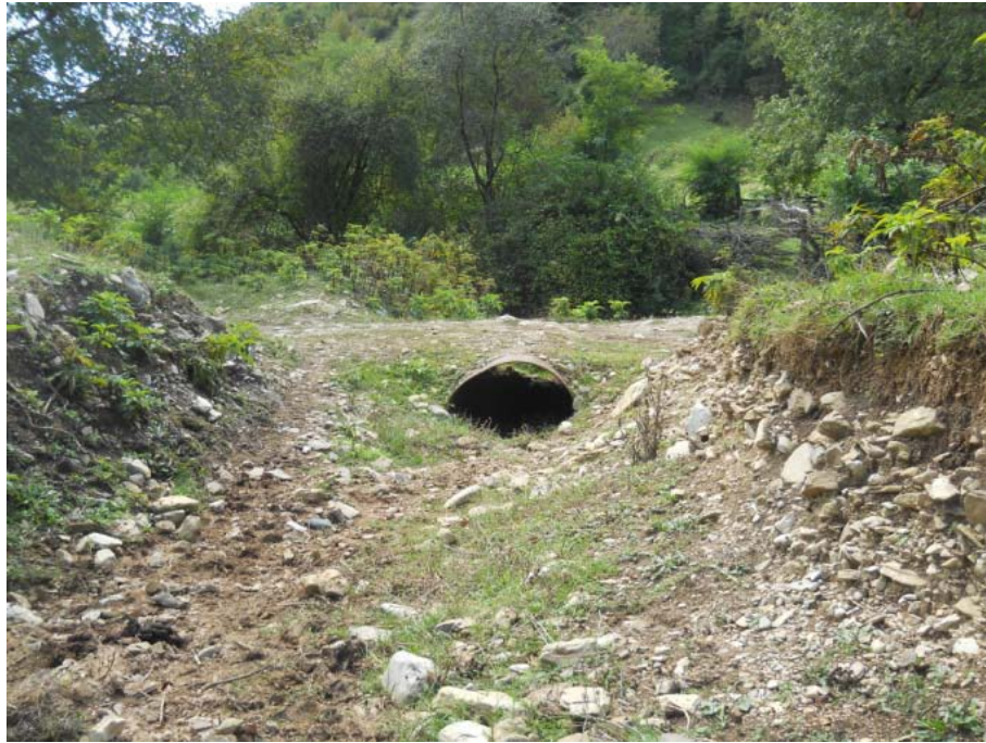
Pic. 14. Pipe bridge at the crossing of the ravine and the motor road
