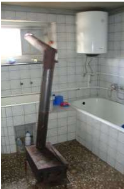
Figure 4.5: Bathroom with an Electric Hot Water Boiler.
