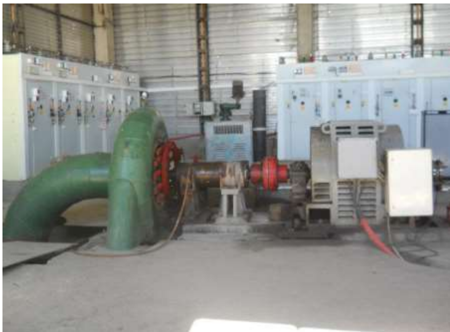
Figure 2.3. Boldoda 0.26 MW HPP, generator
