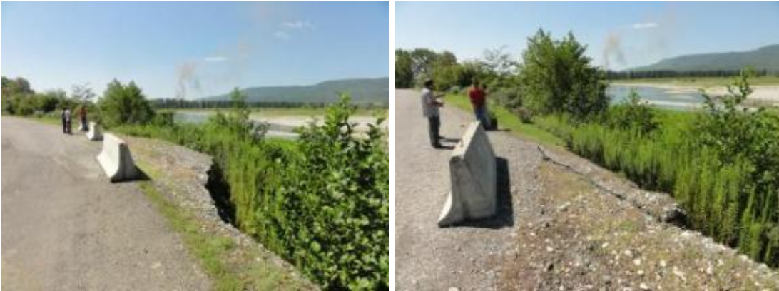
The same process damaged the main bridge on the road connecting Senaki and Martvili. The river has already damaged protective dams of the bridge and one of the supporting pillars.
