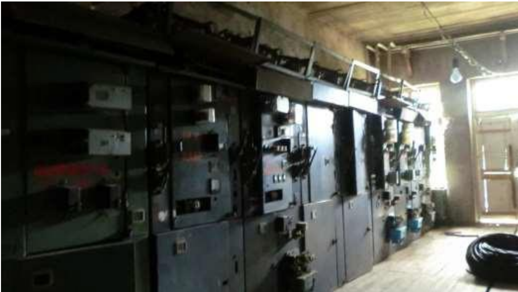
Picture 12-13. Control Board/Operations Panel
