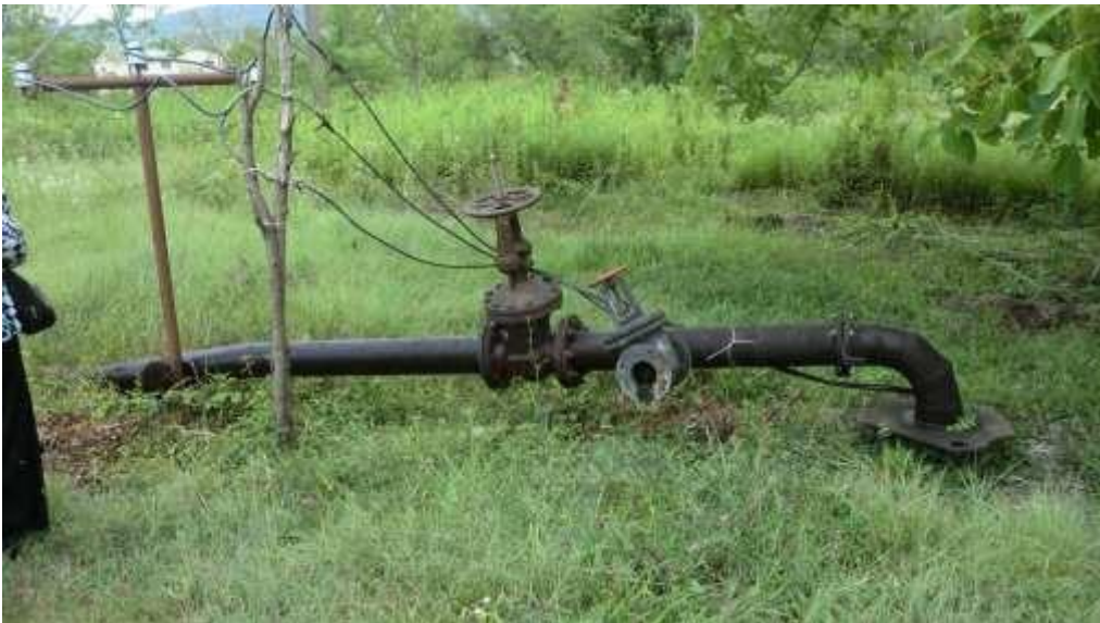
Picture 4. Intake Point of one of the Bore Wells of Nosiri-1 Headworks
