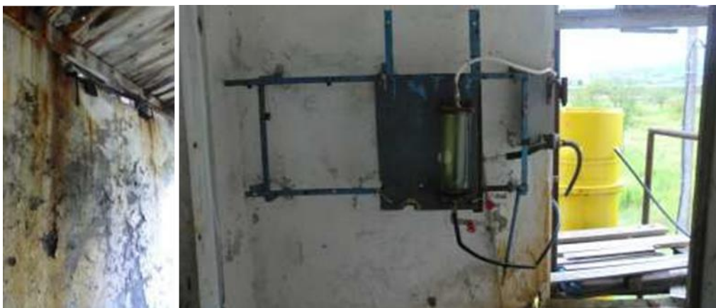
Pictures 6-7. Chlorination Facility and Equipment
