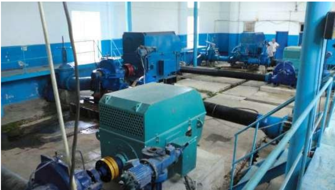
Picture 11. Pump Station with Pumps
