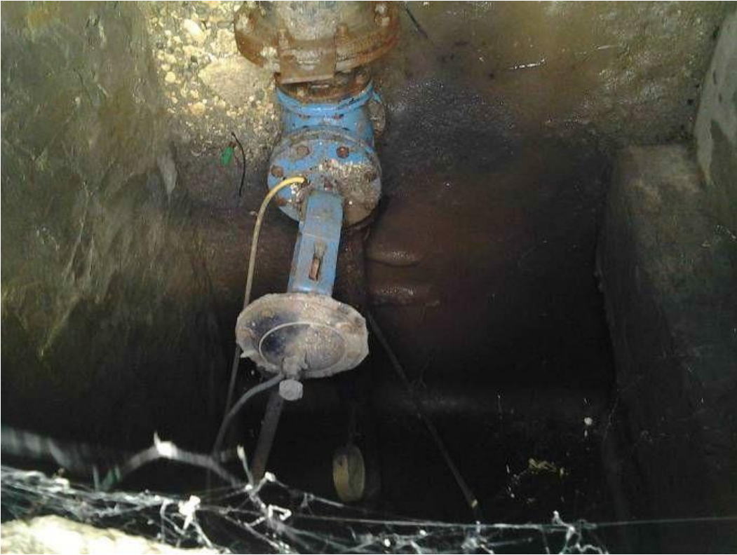
Picture 16. Pressure Control Valve with Manometer
