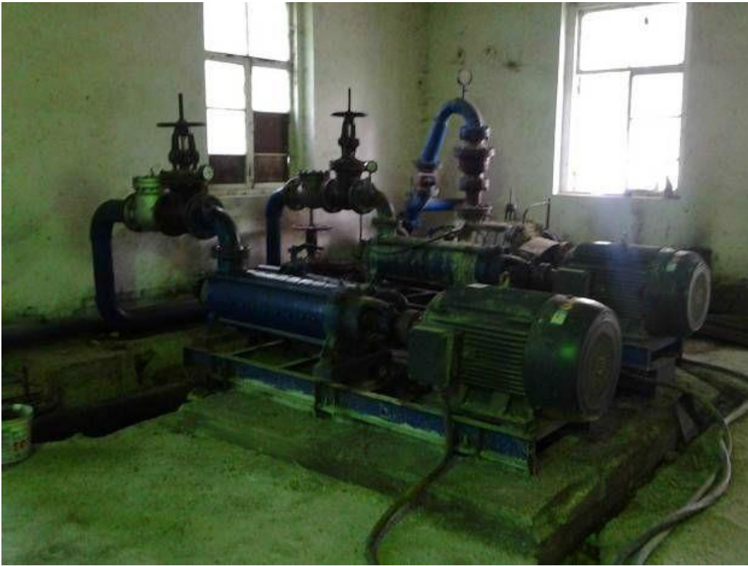
Picture 1. Mazovka Pump Station
