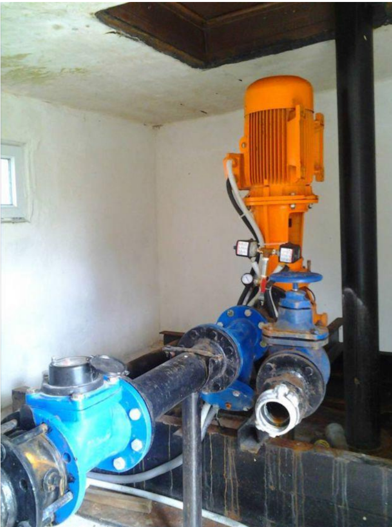
Picture 9. Deep Pump at Stadium Water Collection Well
