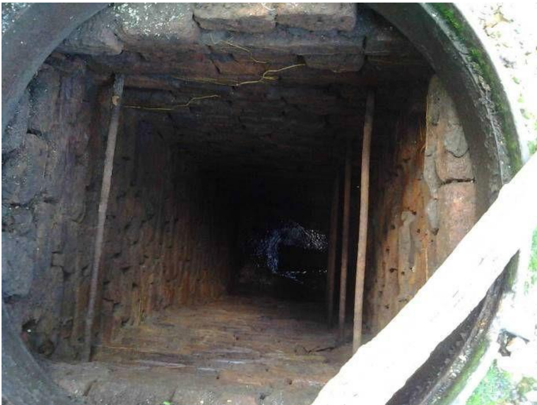
Picture 5.1 and 5.2. Collection Wells at N1 Intake
