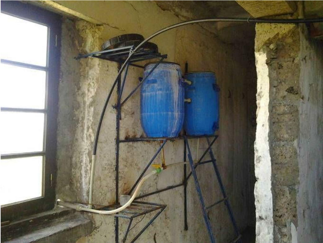
Picture 14. Chlorination Equipment
