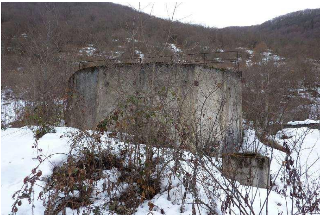
Pic. 5 Settler tank at the headworks “Kvedi”
