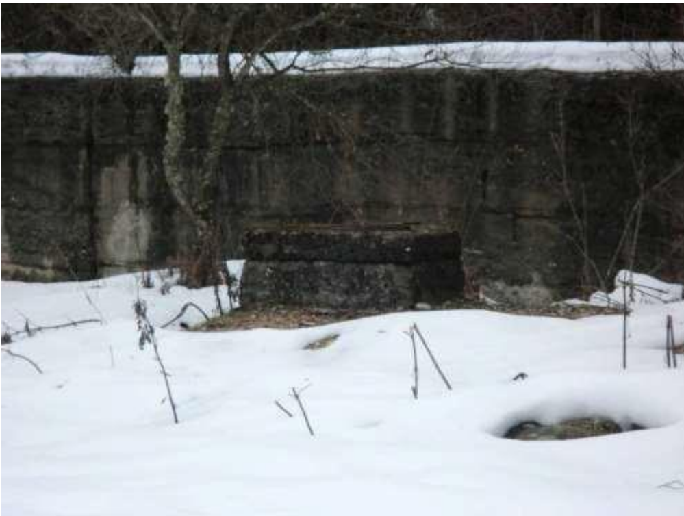
Pic. 4. Destroyed water technological treatment modules at the headworks “Kvedi”
