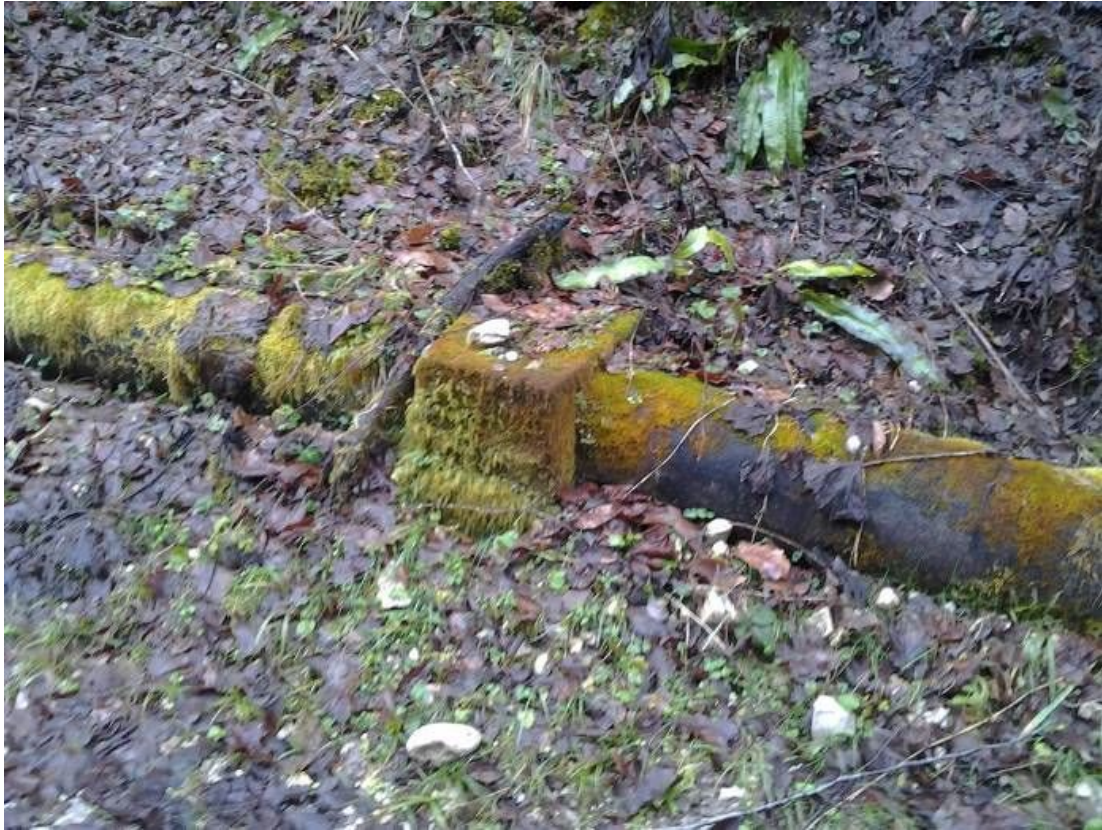
Pic. 6. Water Main Coming from Skhvava Headworks
