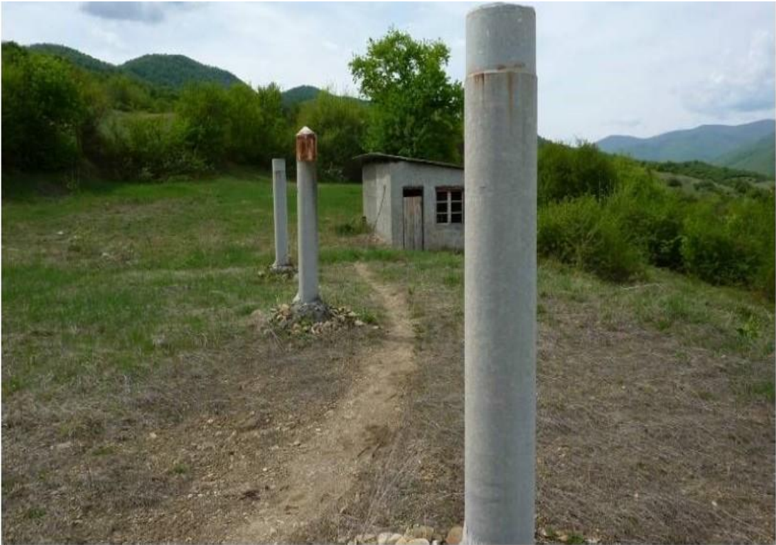
Picture 4&5. Unprotected reservoir roofs and aeration holes
