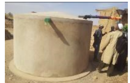
A rain water catchment tank built by USAID WA-WASH in Tiéna (Sahel region).
