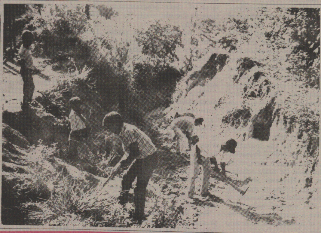
■ The men of Arroyo La Vieja begin work on the roadways leading into the community
