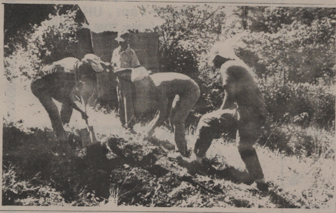
■ The LIFO mission gets underway as work begins on a new latrine.
