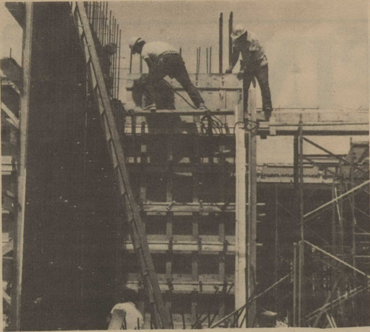
...Despite monsoon type rains that turned the Owa Ehan lot into a new lake, the building is still standing. Workers are seen here trimming the wood on the first floor of the new building expected to be ready by next year.
