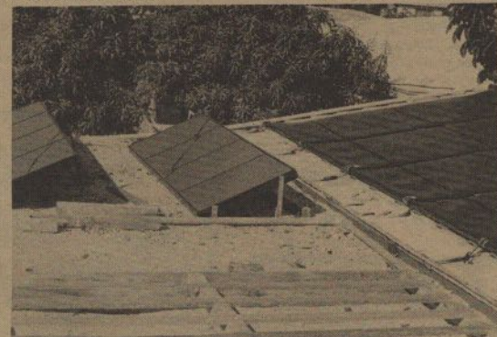
CAPITAL AND SOLAR-FAFRO PANELS
