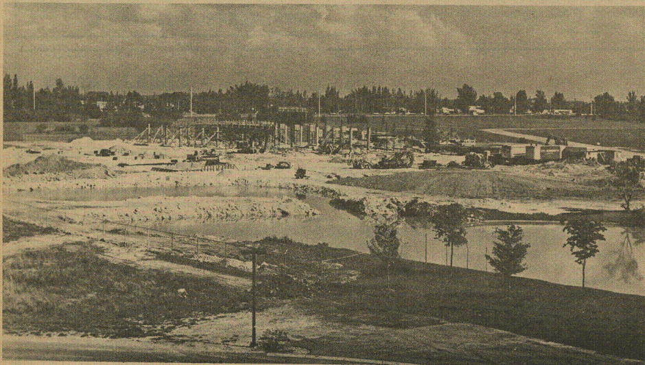
Construction on buildings four and five make the flat landscape rise with steel girders and cement blocks as crews are underway, developing the next structures at
