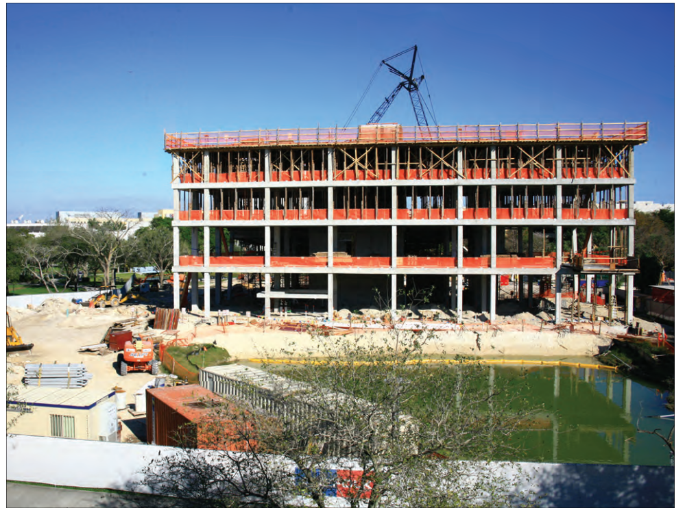
Construction of the new building for School of International and Public Affairs began last year and is expected to be completed this November. The building has a proposed silver LEED certification, in part due to 3 percent of the building’s energy coming from the roof’s solar panels, in addition to a green roof.
