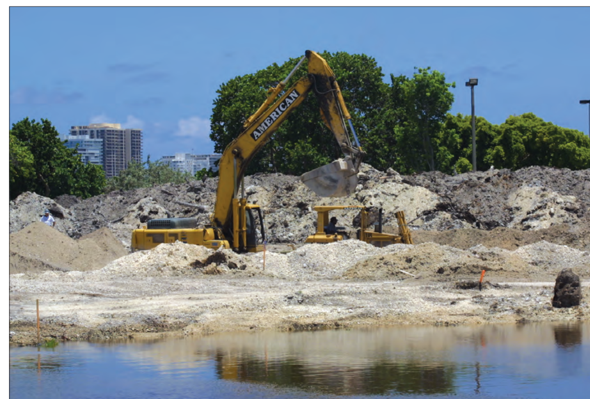
BREAKING GROUND: An excavator digs up and removes dirt from the future site of the new Marine Biology building to be located near the Wolfe University Center at the Biscayne Bay Campus. Construction on the site began after the groundbreaking ceremony held on April 23. The new waterfront marine building will allow students and faculty to work in 57,000 square foot laboratory. ALFREDO SOTO/THE BEACON
