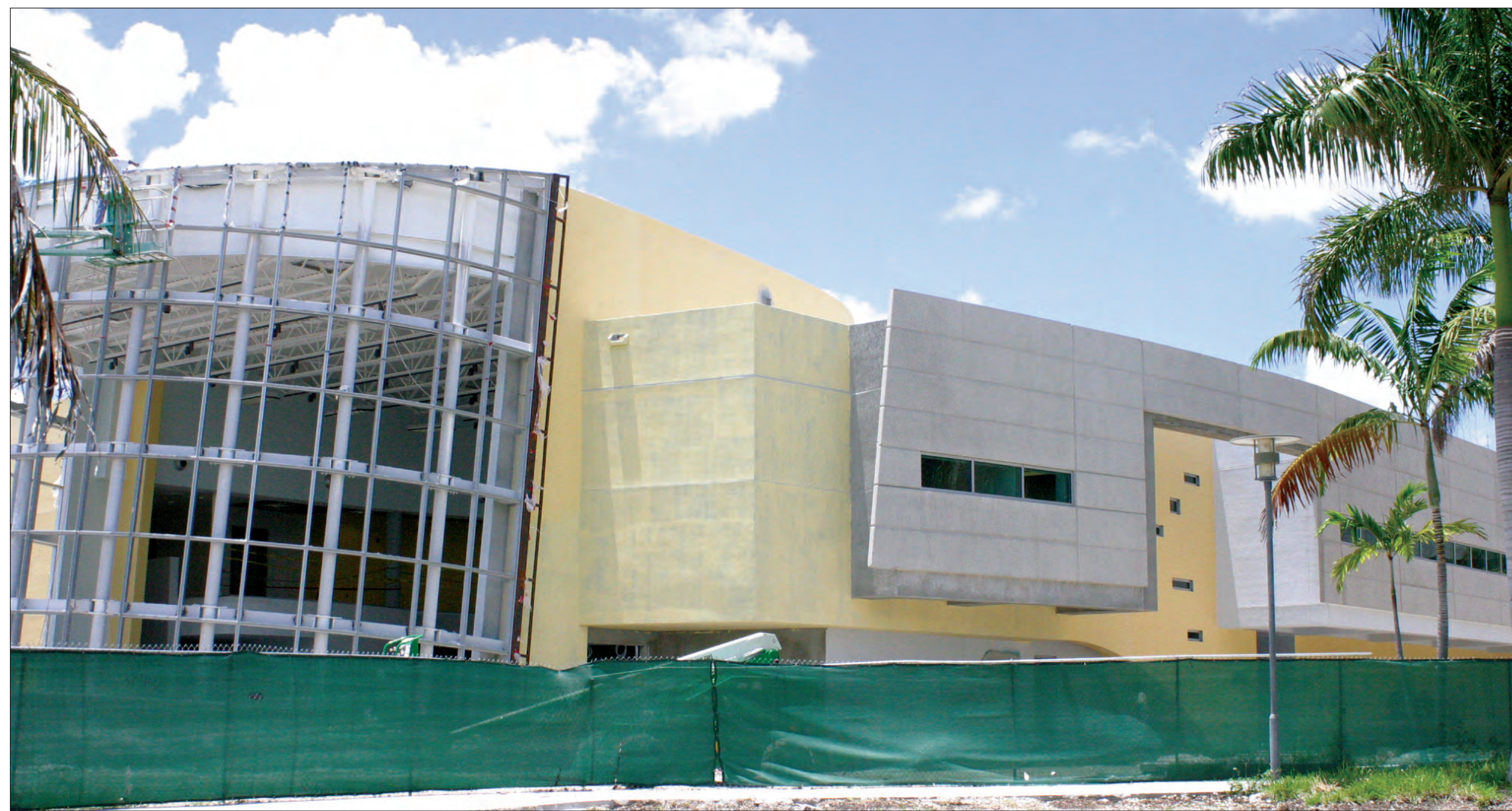
FACE LIFT: As part of continuing construction, the Graham Center is receiving a major facelift. Glass panes will cover the enormous steel skeleton (above) and become a new back entrance that is sure to turn heads. An additional renovation includes a new wing which features a beautifully designed outside wall facing the Green Library. EMILY JENSEN/THE BEACON
