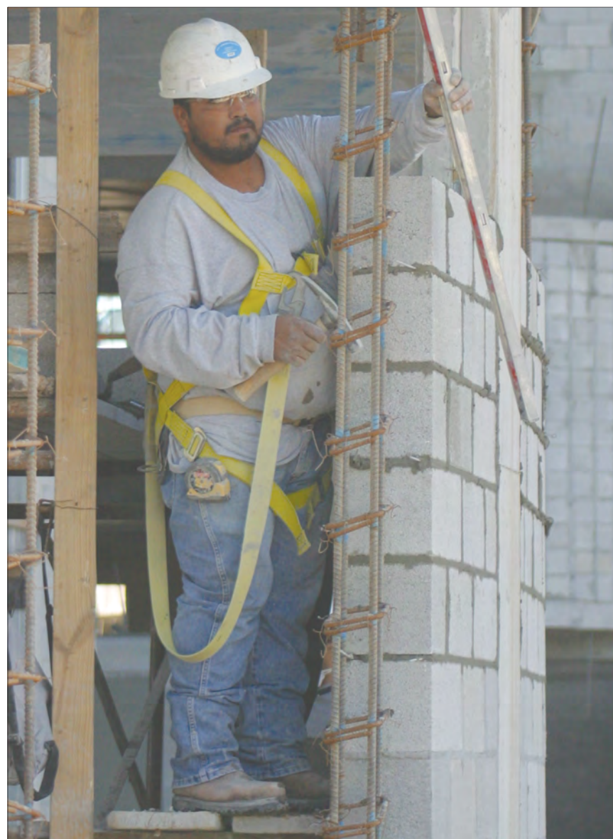
BUILDING IT: Mason Francisco Rodriguez works on a wall of the new Lakeview Hall which despite hurricanes, is still scheduled to open for Fall 2006. Sign up begins Feb. 27. HARRY COLEMAN/THE BEACON
