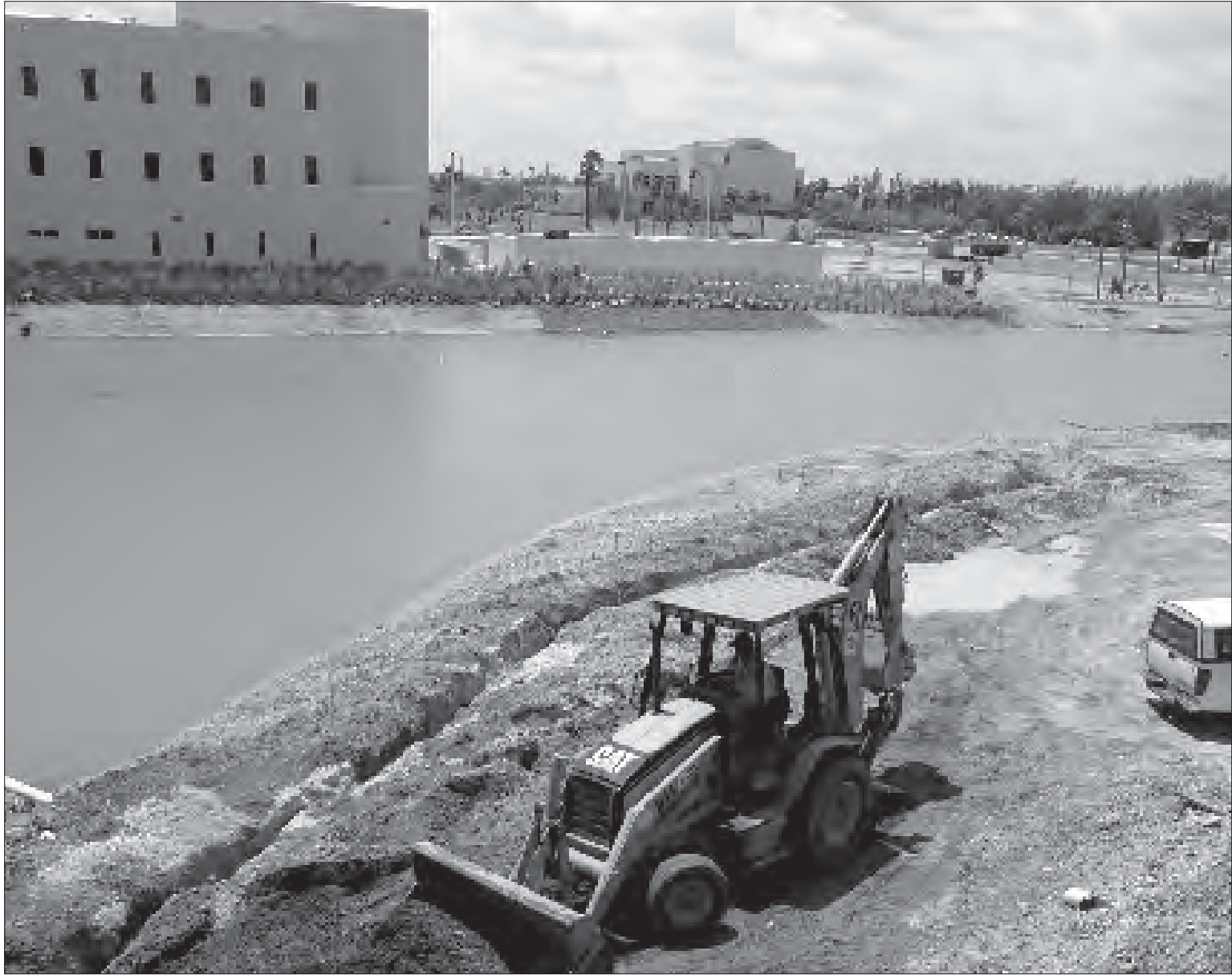
ALMOST THERE: Administrators at the Biscayne Bay Campus anticipate that construction crews at the marine biology site will be gathering its tools and exiting by the end of the month. MARISA FIALHO/THE BEACON
