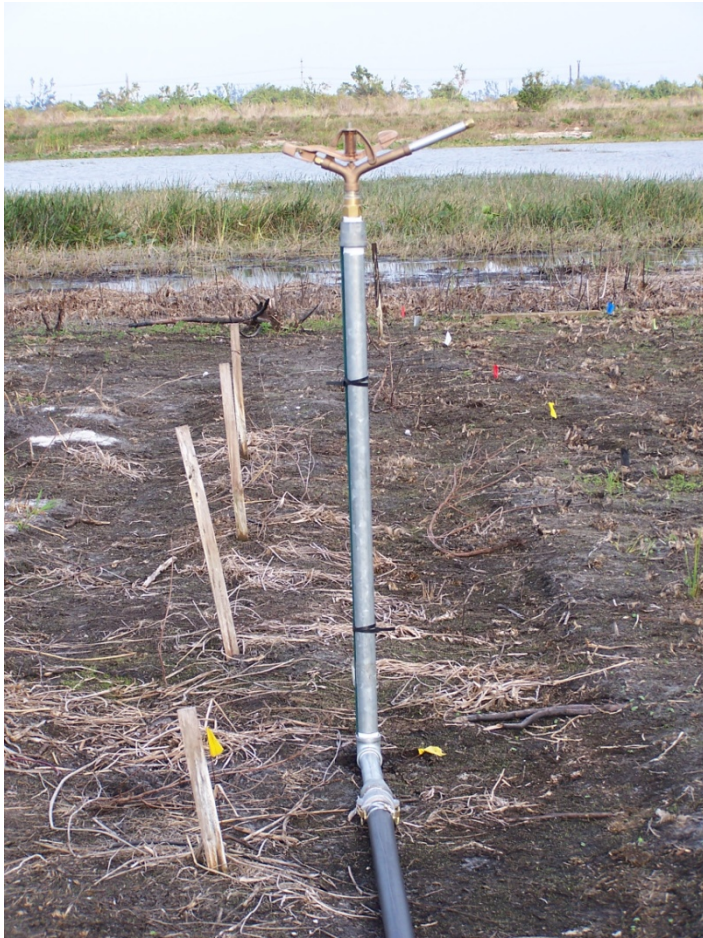
Figure 4.1 and 4.2. Irrigation system on one of the tree islands showing t-valve (top) that diverts water to each of the 2 standpipes and nozzles on each tree island (bottom) as required to partially satisfy Task 2a.
