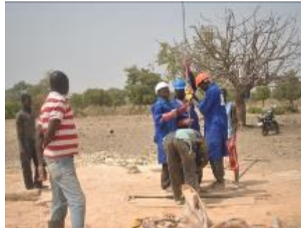
A team of manual drillers at work in the village of Vipalgo, Burkina Faso.
