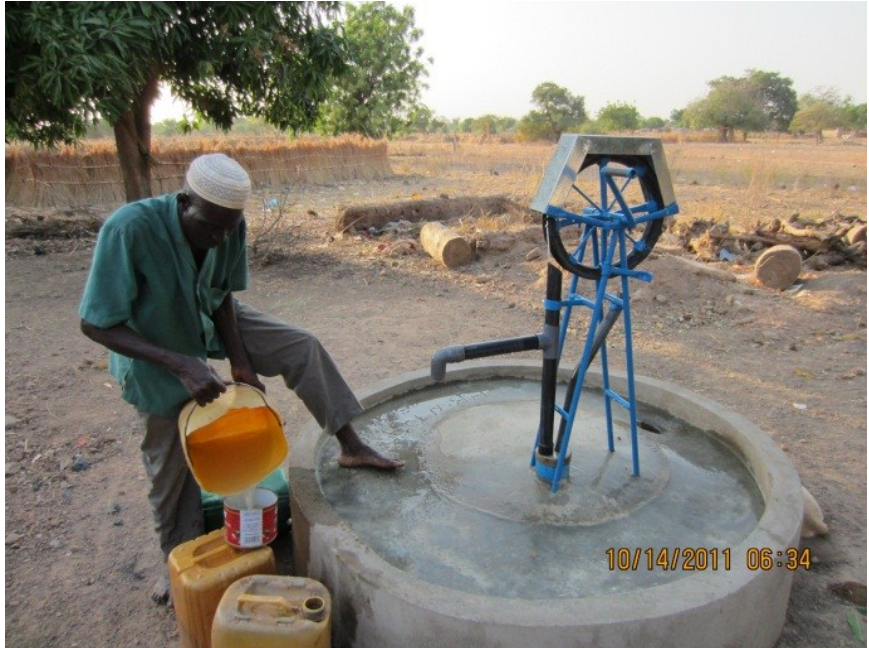
A rope pump installed in Oueglega
