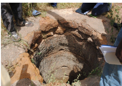
A traditional well that has collapsed in Oueglega
