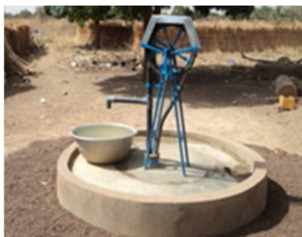
A rope pump installed in the village of Oueglega
