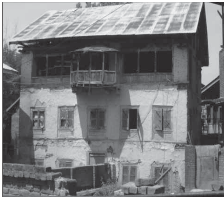
Figure 1. Houses with typical Taq type construction in Srinagar. Photo: Amir Ali Khan
