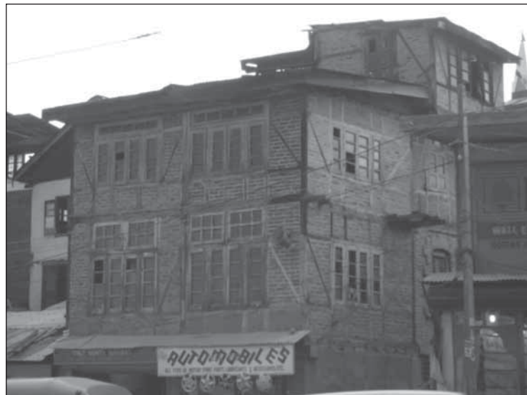
Figure 2. Houses with typical Dhajji-Dewari system of construction in Srinagar. Photo: Amir Ali Khan
